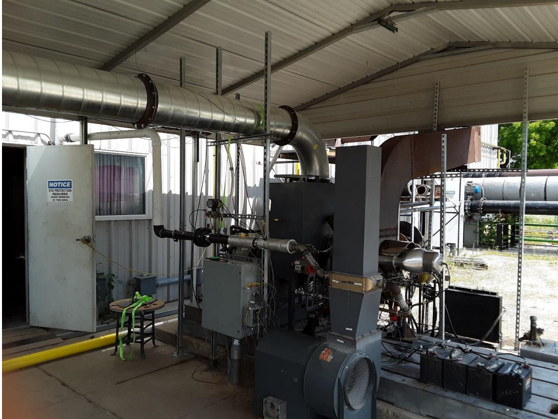
Figure 2. Allison 250 C28B engine test facility
