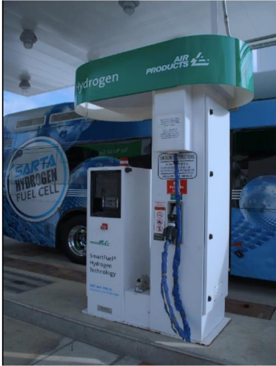
Figure 9. Hydrogen Fuel Station
