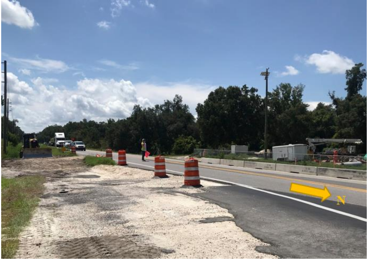
Figure 44. Flag Operation and Queue Formed in Phase 4B1 at US-98 and Trilby Rd
