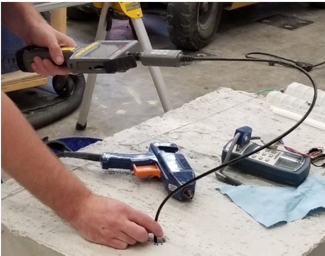
Figure 17. Photo. Insertion of borescope to verify correct placement of duct bonding glue.
