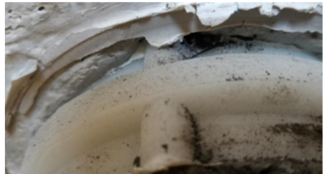
(b) Photo. Traces of grout on outside of duct, which resulted in low AC impedance readings.
