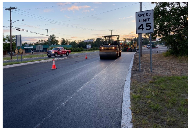
NJDOT treated more than 900 miles of roadway with HPTO between 2008 and 2018. Source: NJDOT
