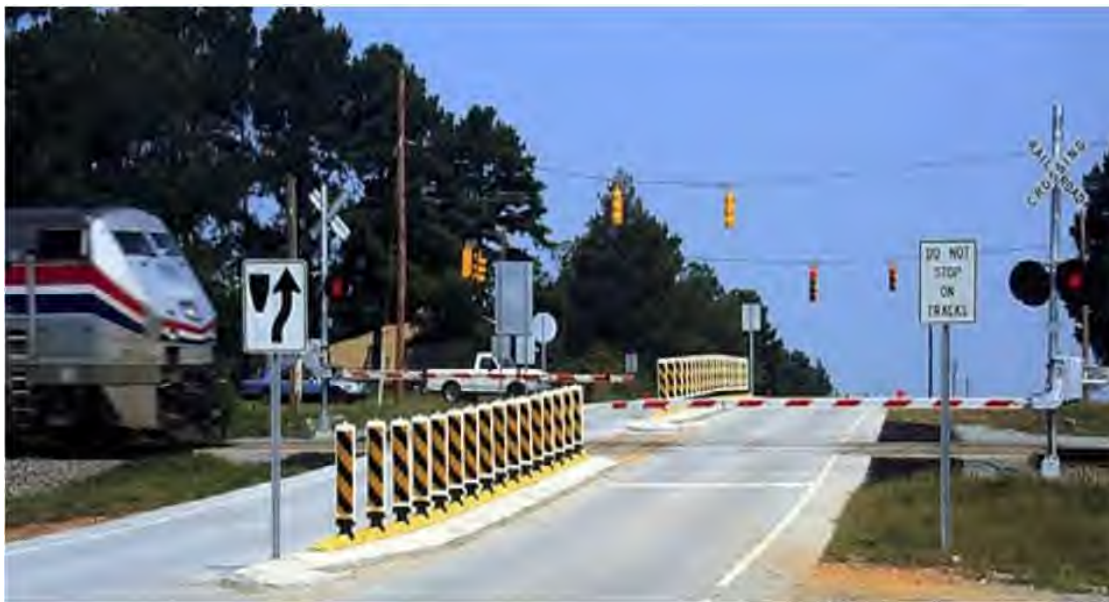
Figure 56 An example of a mountable raised curb system. Source: U.S. DOT. (2019). Highway-Rail Crossing Handbook (Figure 37)
