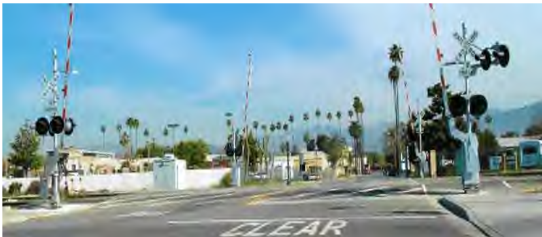
Figure 45 An example of four-quad gates. Source: FDOT. (2013). Improved Traffic Control Measures to Prevent Incorrect Turns at Highway-Rail Grade Crossings (Figure 2-21)
