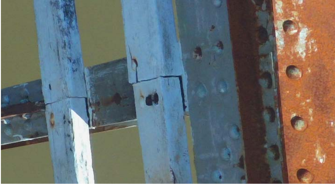
Figure 43. Photo enlargement of another section of the bridge superstructure shown from the inside deck, view, showing the condition rail with apparent crack near rivet.
