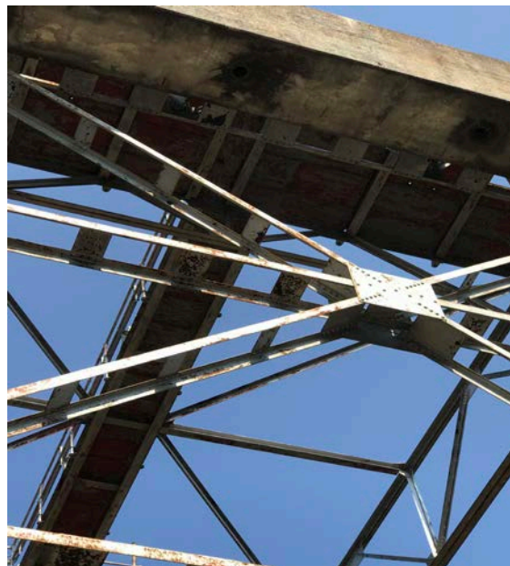
Figure 22. Shows a close up of the bridge superstructure top section showing tight spaces between structural members.
