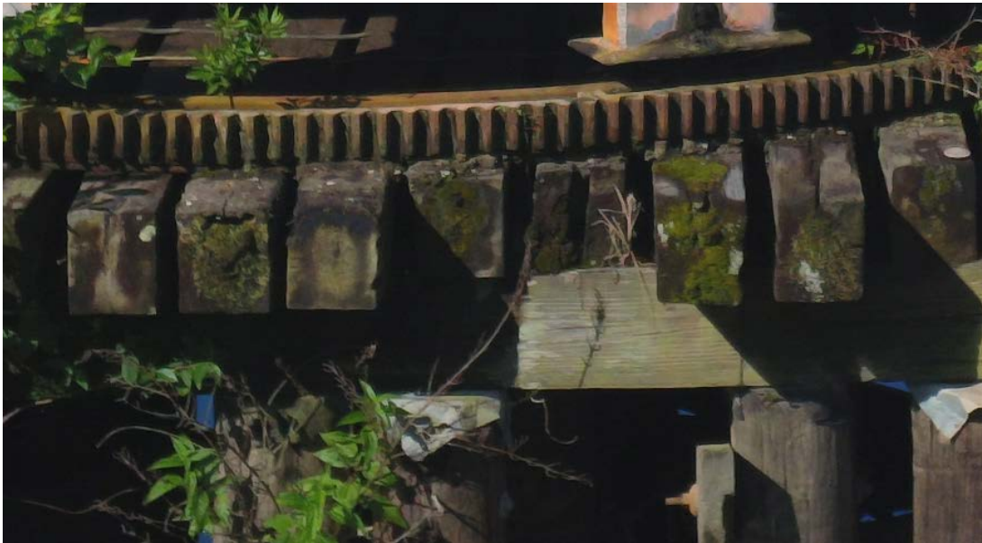
Figure 44. Photo enlargement of timbers supporting the entire bridge swing mechanism, showing apparent exterior wood decay.
