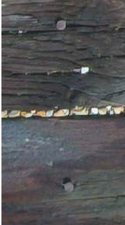
Figure 41. Photo enlargement even closer of another section of the bridge deck, showing board cracks and protruding nail heads.
