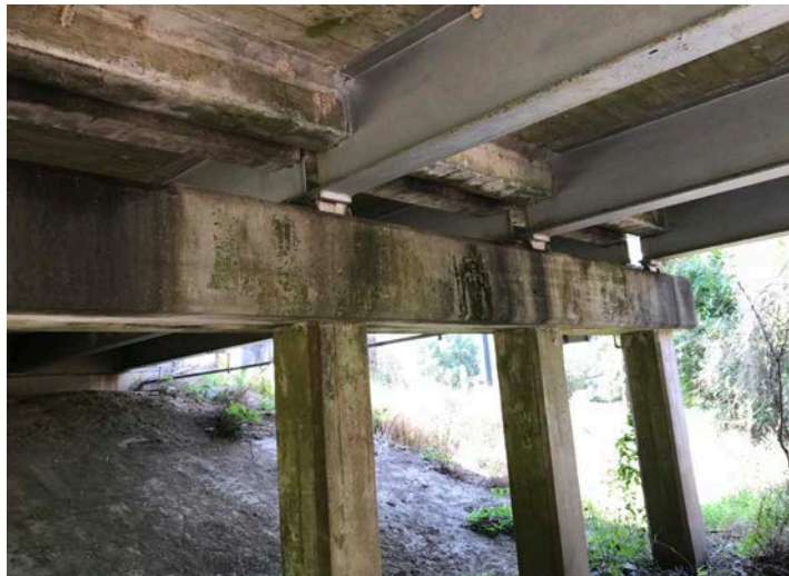
Figure 24. Again shows tight space confinement beneath the deck of the sample bridge.
