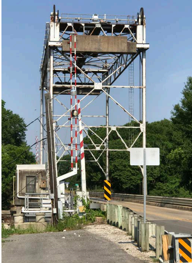
Figure 21. Shows an overview of the Vermilion River Bridge in Milton, LA, i.e. the sample bridge.
