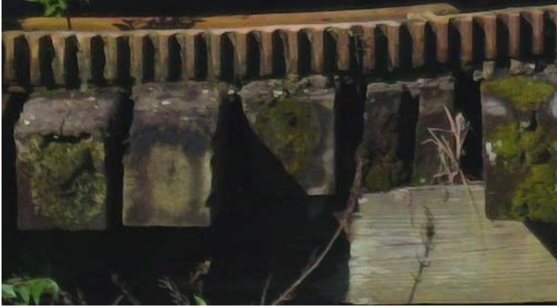
Figure 45. Further enlarged image from Figure 44, showing close view of the affected support timbers.
