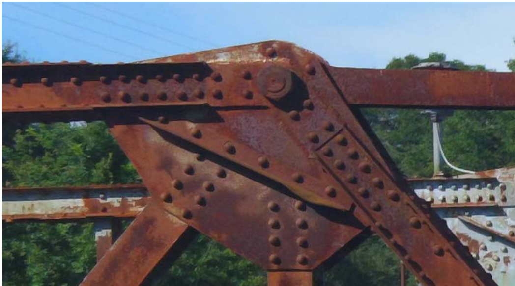
Figure 36. Photo enlargement showing the condition of joint and rivets in the northeast side of the bridge superstructure truss.
