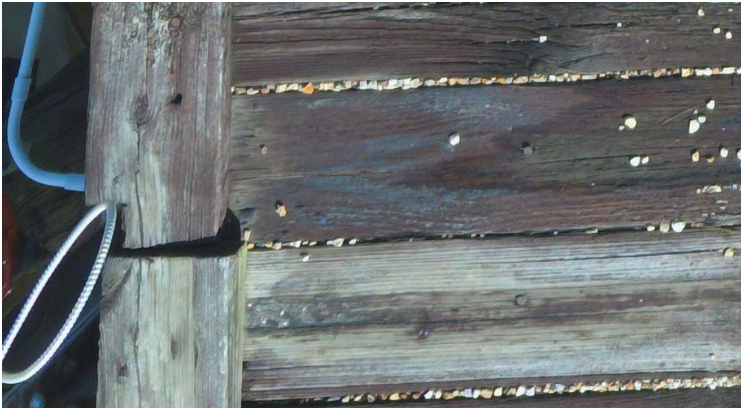
Figure 40. Photo enlargement of another section of the bridge deck, showing the condition bridge deck boards shown from top, where apparent board misalignment is seen as are the heads of protruding nails.
