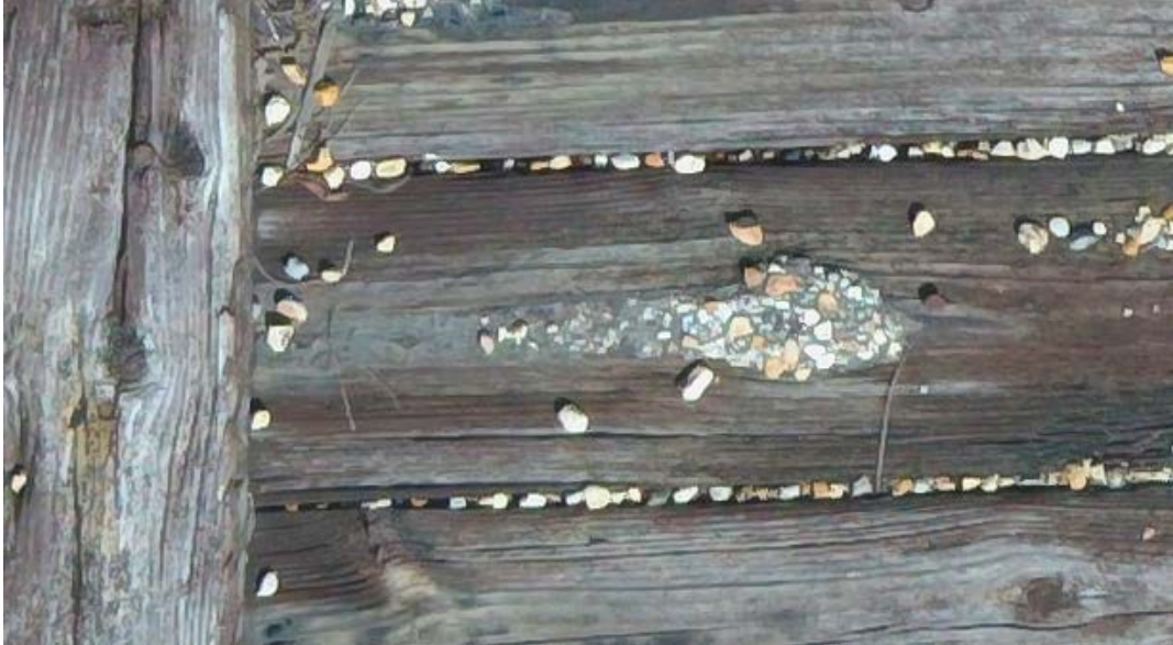
Figure 39. Photo enlargement showing the condition bridge deck boards shown from top, where cracks in the exterior of deck beam are visible as are nail heads slightly protruding from the deck board.
