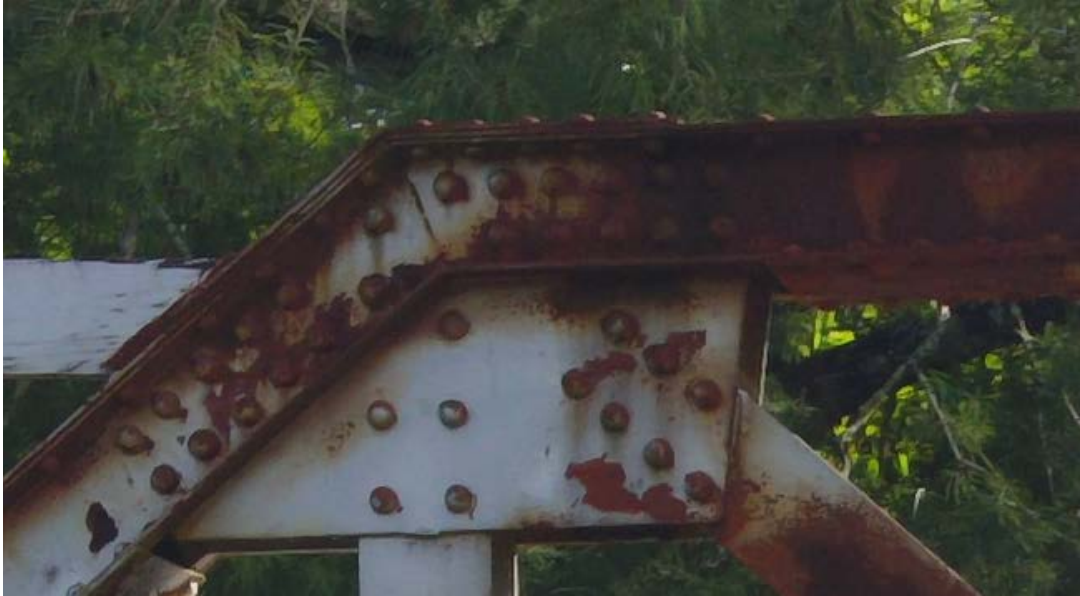
Figure 33. Photo enlargement showing the condition of bridge superstructure joint and outside rivets.
