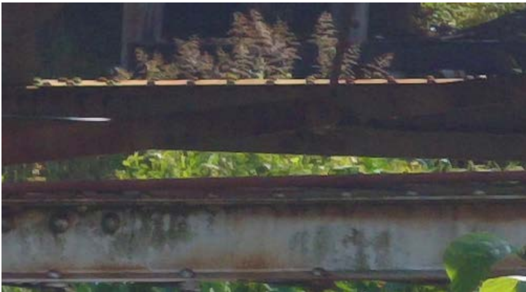
Figure 34. Photo enlargement showing the condition of the near and far rivets in the lower members of the superstructure truss.
