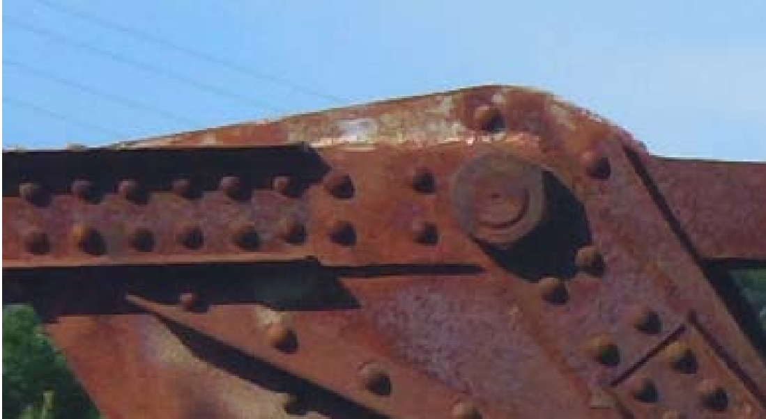
Figure 37. Photo – greater enlargement of same joint shown in Figure 36, again showing closer snapshot the condition of joint and rivets in the northeast side of the bridge superstructure truss.
