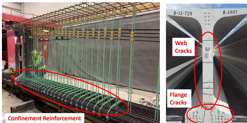
Figure 36 - Girder reinforcement prior to casting concrete (left) and representative end cracking (right).
