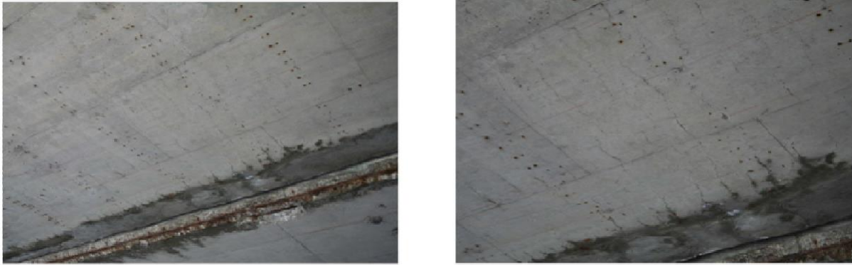
Figure 2 - Examples of under deck bridge cracking. Photos are from a previous WHRP report [5].
