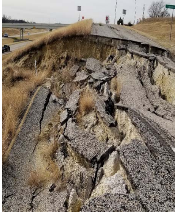
Figure 11. Texas site observed height of slope failure.
