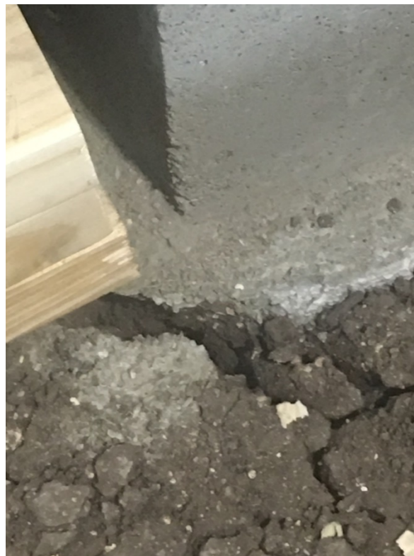
Figure 32. Surface cracking during testing.
