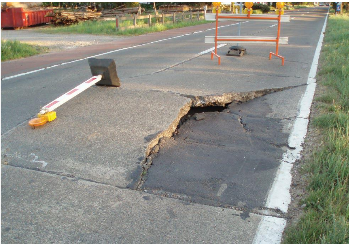
Figure 45. Buckling caused by HMA patching (Rens 2018).
