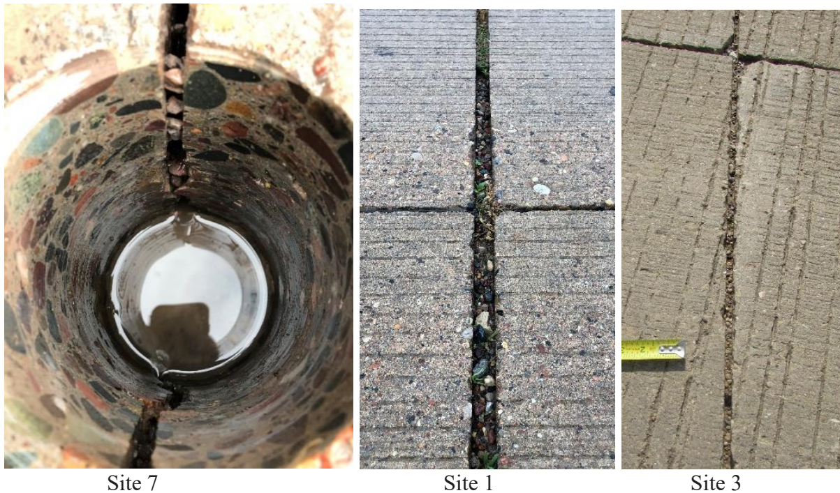
Figure 22. Photo of incompressibles in the transverse joint.
