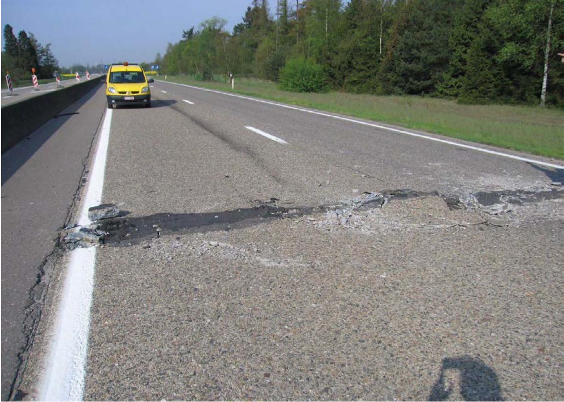
Figure 46. Buckling caused by poor joint sealing (Rens 2018).
