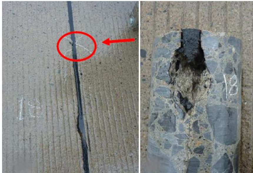
Figure 66. Deterioration below the surface of a visibly intact joint on Hwy 417 (Chan et al. 2020).
