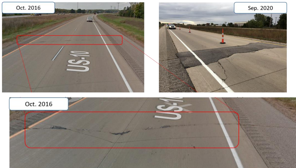
Figure 13. Google Earth® images of U.S. 10 in Portage county (site # 1) prior to buckling showing spalls, shoulder cracking, and asphalt patching (left and bottom). Image on the right, collected during the September 2020 field survey shows the same location patched with full-depth asphalt following the blowup.
