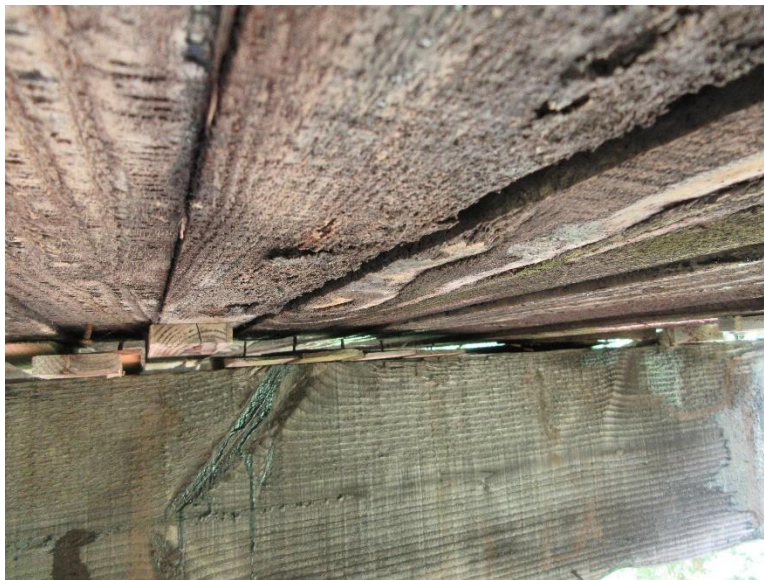
Figure 4-52 Missing shims or gapping between spreader beam and bottom side of deck (La Crosse Co. P320083)
