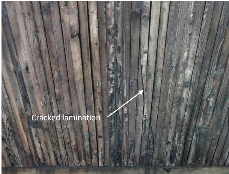
Figure 4-54 Cracked Lamination (La Crosse Co. P320083)
