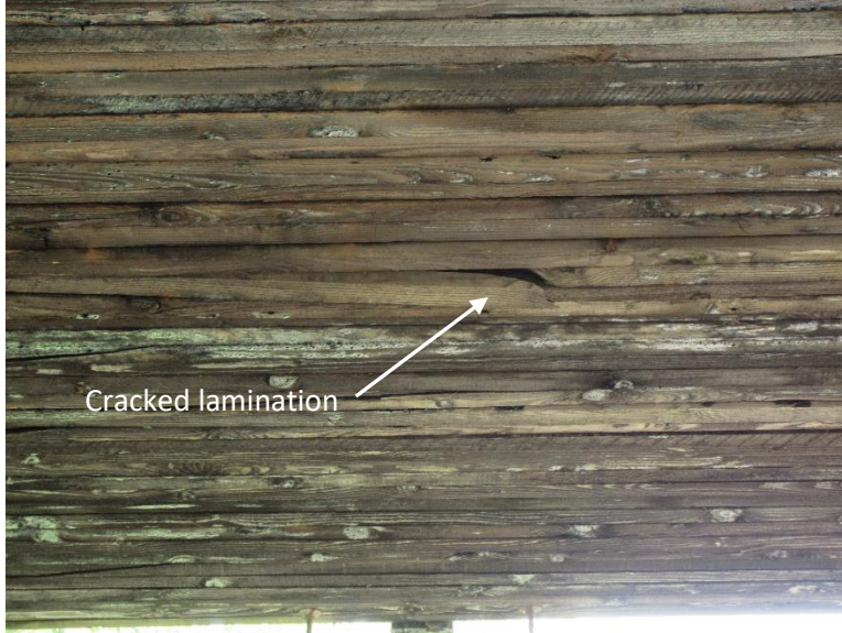
Figure 4-53 Cracked Lamination (La Crosse Co. P320083)
