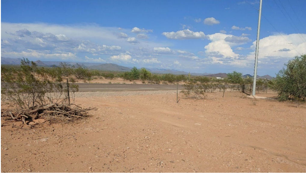
Figure 57. ROW Fence Cut to Access a Nearby OHV Trail
