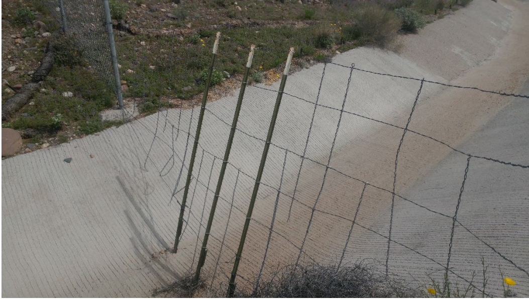
Figure 60. Section of Barbed Wire Fence Within a Chain-Link ROW Fence to Bridge a Drainage Feature
