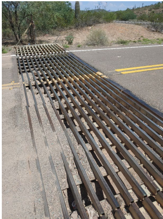
Figure 63. Crossing Guard with More Than 50 Percent Sedimentation
