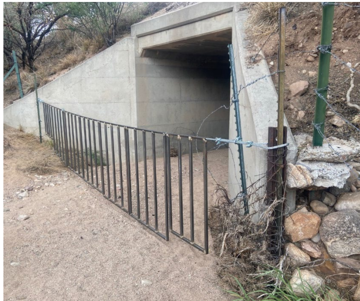
Figure 71. Swinging Gate Design to Prevent Burro Passage But Allow Hydrological Flows
