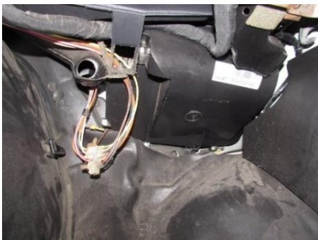
View of HVAC from interior
