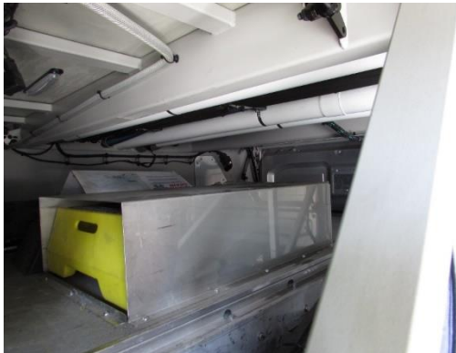
View toward rear of cable routing
