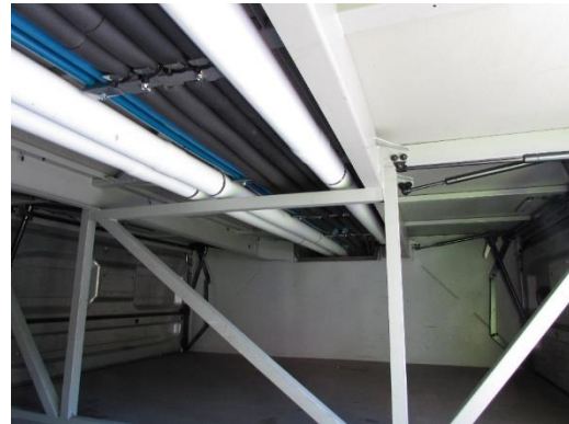
View toward front of cable routing
