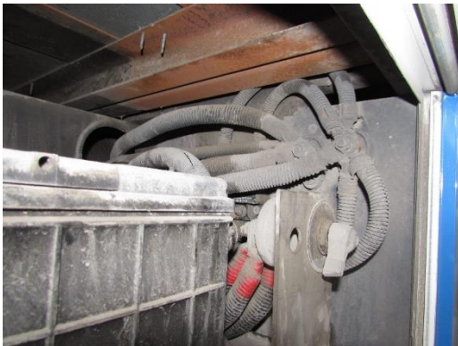
Additional view of battery cable routing
