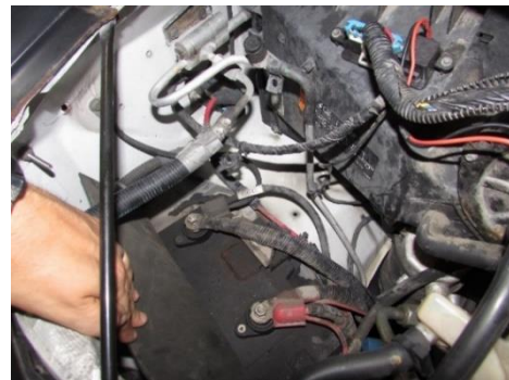
Showing battery under/adjacent HVAC
