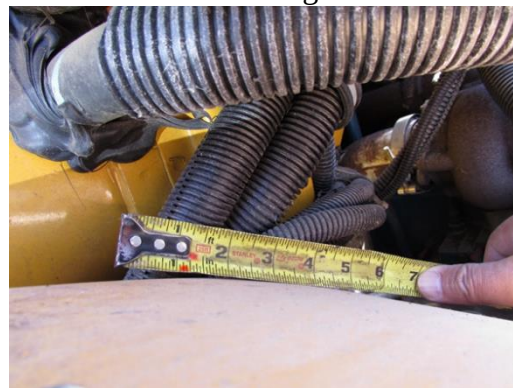
Firewall on left side (close-up view)
