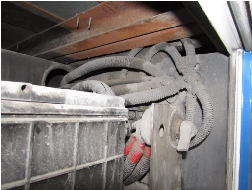
Additional view of battery cable routing
