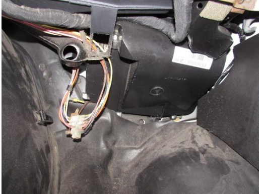
View of HVAC from interior
