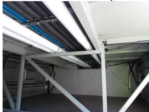
Cable routing through luggage area
