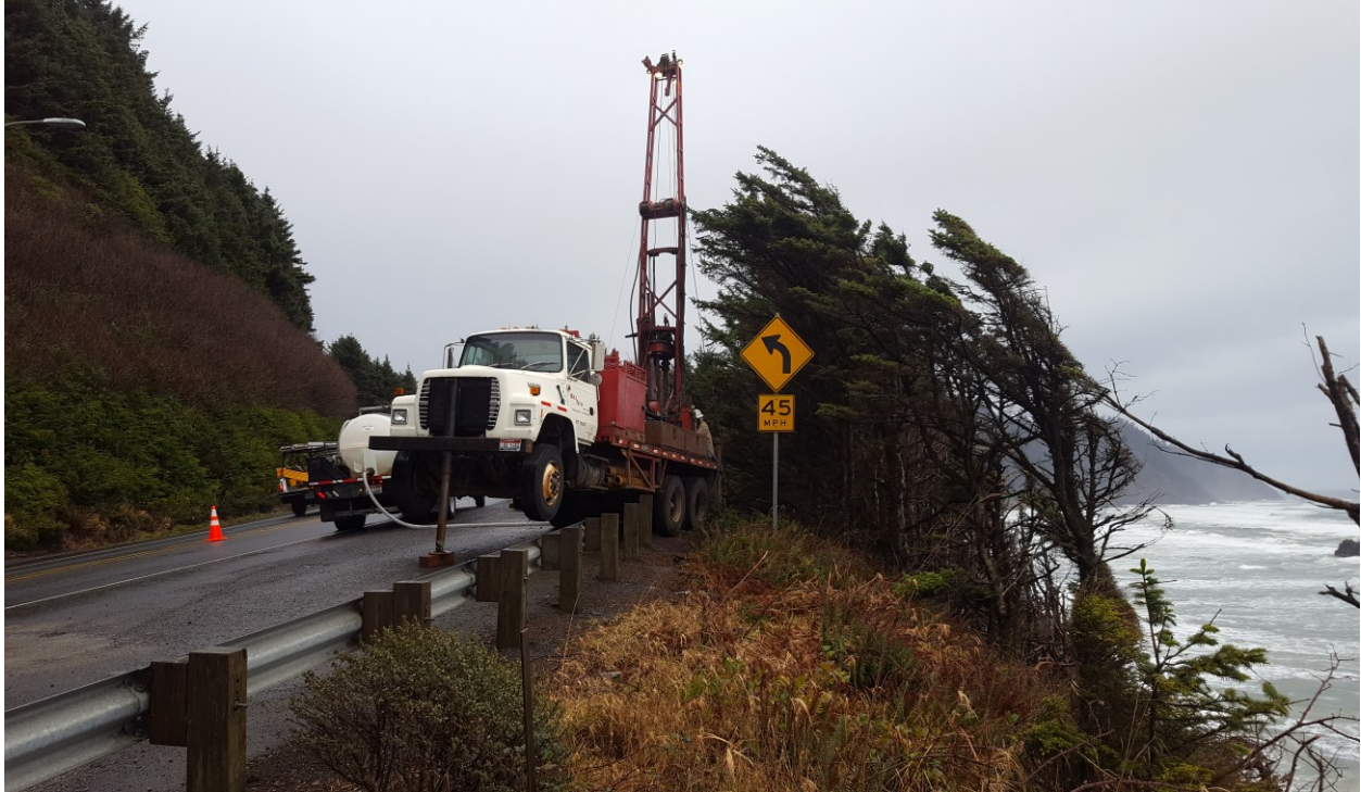
Figure 2.10: Drill rig actively drilling borehole for SAA MEM's installation at Arch Cape on January 20, 2017. Photograph Credit: Dr Michael Bunn.
