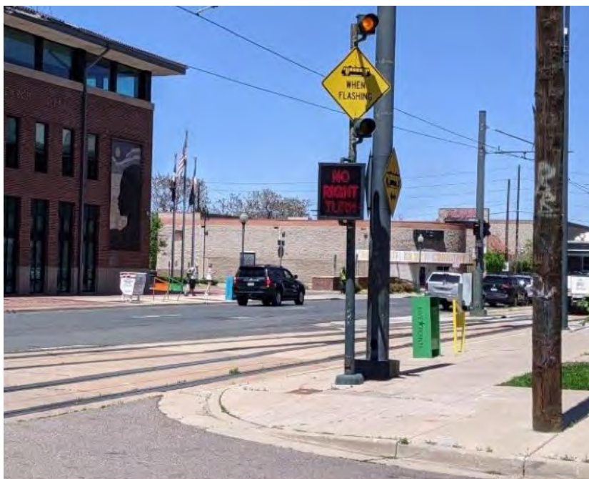
Figure 6-53 Dynamic “No Right Turn” sign and flashing lights activated at intersection on L Line
