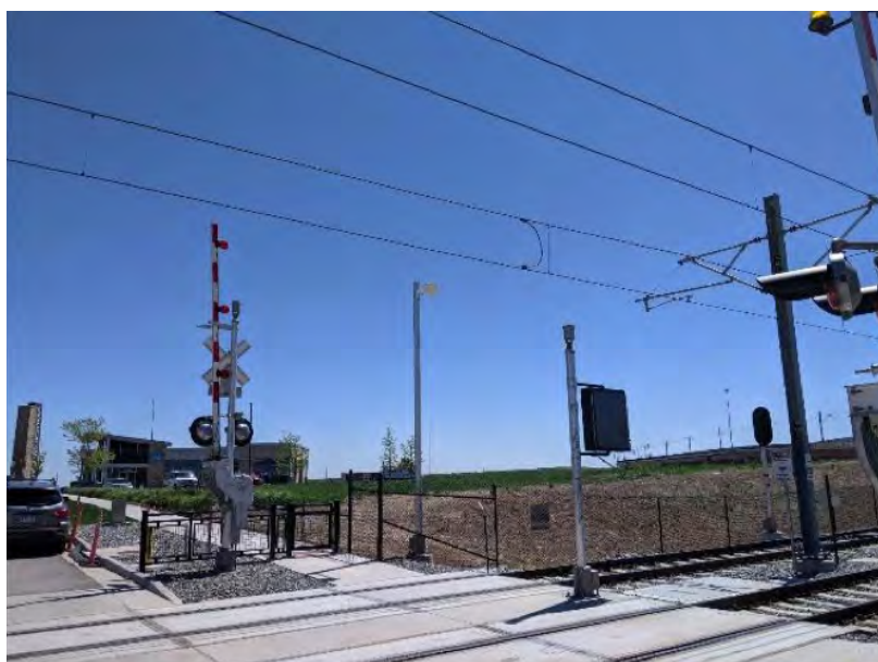
Figure 6-70 Grade Crossing at Sky Ridge Station; sensor for occupancy detection system on pole on far side
