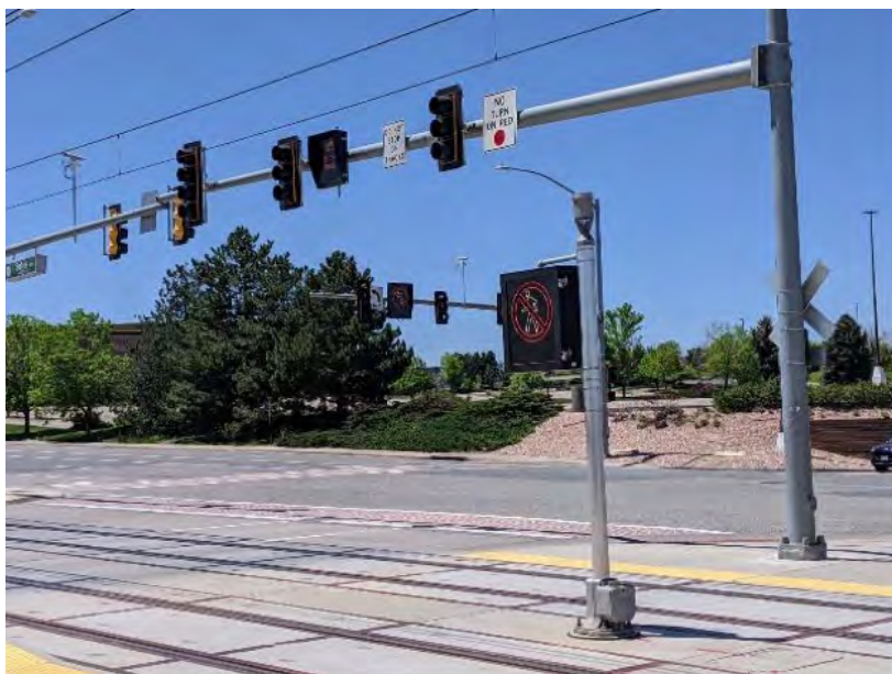
Figure 6-79 Grade crossing protection by traffic signals, plus two dynamic signs for motorists, one more for pedestrians
