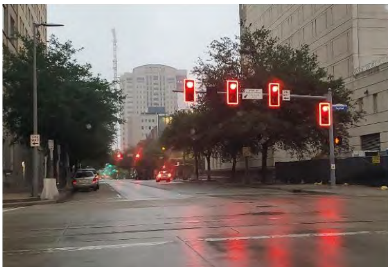
Figure 6-8 Illuminated LED borders on red phase of traffic signal protecting against rail movements; note use of mast arm to accommodate additional signal heads
