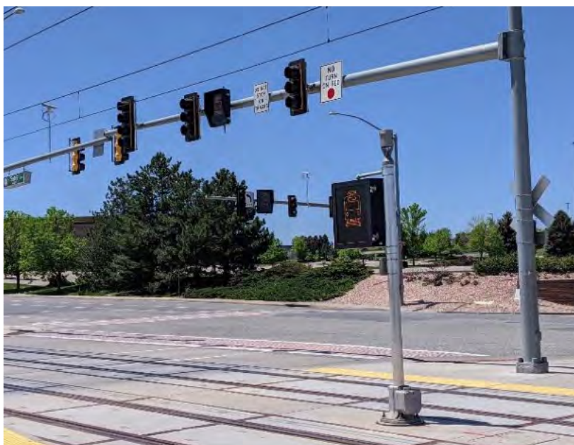
Figure 6-80 Grade crossing protection by traffic signals plus two dynamic signs for motorists, one more for pedestrians; dynamic sign for pedestrians alternates between “Do No Cross” and “Train” warning
