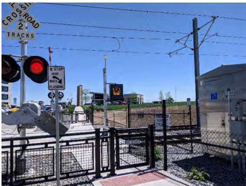
Figure 6-67 Grade Crossing at Sky Ridge Station; note pedestrian swing gates, sidewalk pavement treatment, signage, dynamic sign
