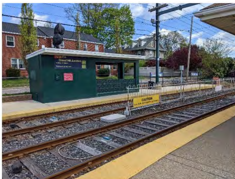
Figure 6-115 Rail vehicle detection equipment in track near grade crossing
