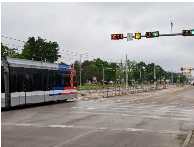
Figure 6-5 Dynamic sign indicating approaching train for left-turn-only lane
