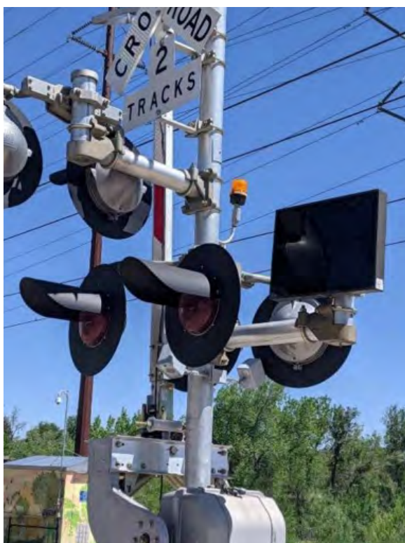
Figure 6-62 Typical crossing on West Line; amber beacon indicates crossing activation to train operators
