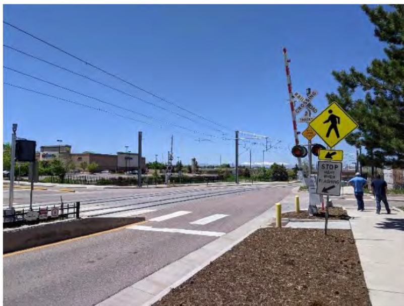
Figure 6-87 Grade crossing and track transition at northwest corner of R Line diversion, westward view
