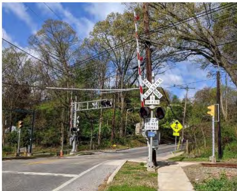
Figure 6-117 Conventional grade crossing equipment at one crossing on single-track portion of Media Line; bar signals for rail traffic also used
