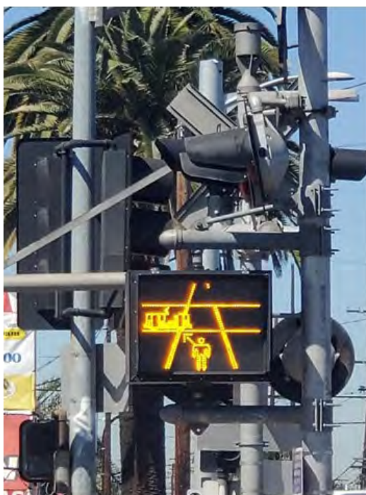
Figure 6-23 Dynamic sign warning pedestrians of trains on two tracks – look left indication
