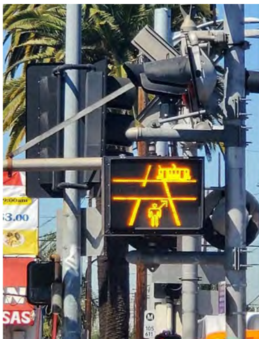
Figure 6-22 Dynamic sign warning pedestrians of trains on two tracks – look right indication
