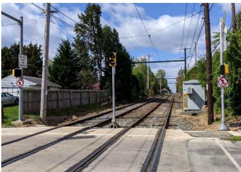
Figure 6-110 View looking across street showing bar signal and “Do Not Walk” signs
