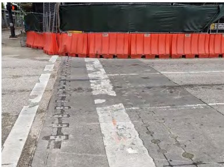
Figure 6-10 Remains of in-pavement lighting system that suffered frequent failures, required high maintenance
