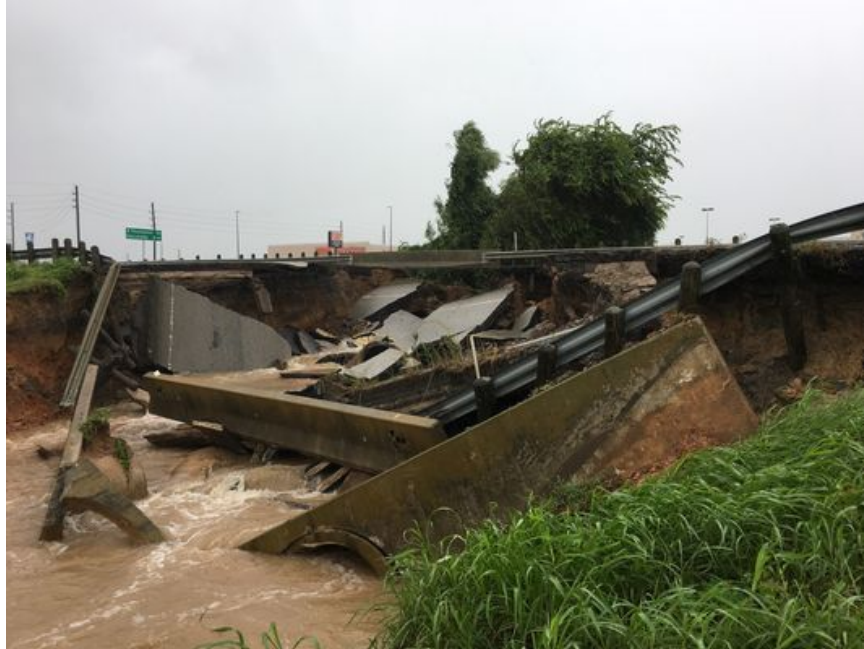
Figure 1. Bridge Collapse near Rosenberg TX as a result of Hurricane Harvey (2).
