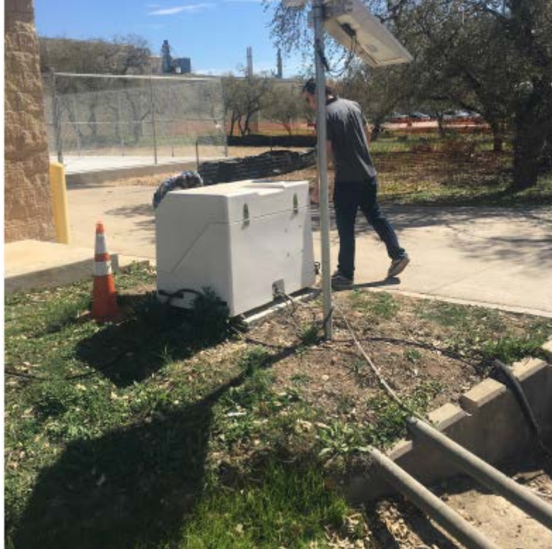
Figure 21. Control box of the Signature flowmeter installed on campus.
