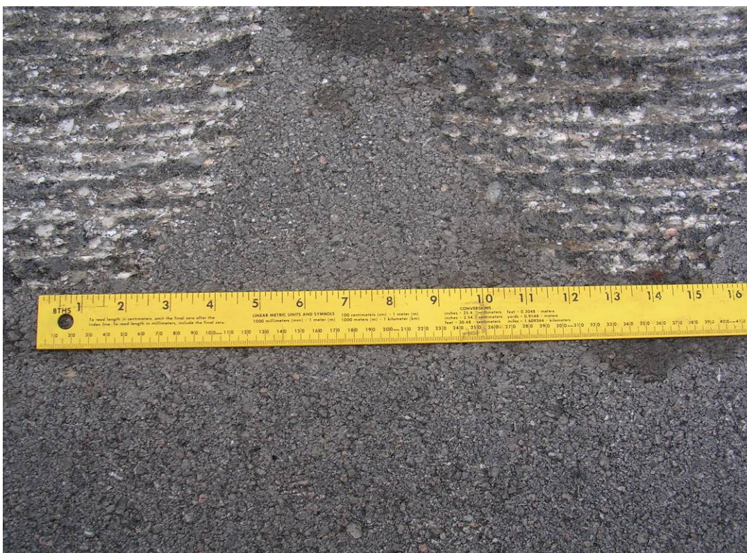
Figure A3: Distance between football rumble strips center-to-center (approx. 14 in.)
