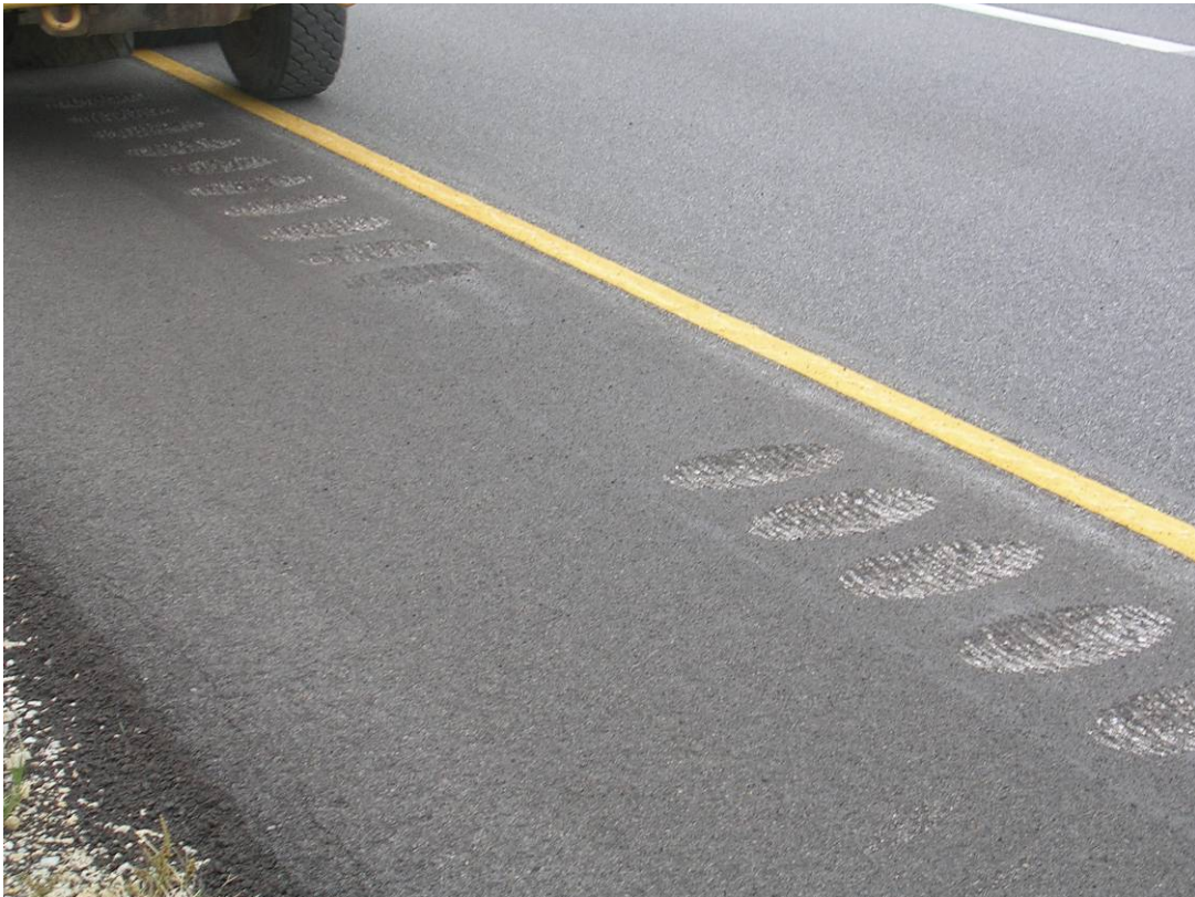
Figure A7: Football shaped rumble strips after clearing of milled debris
