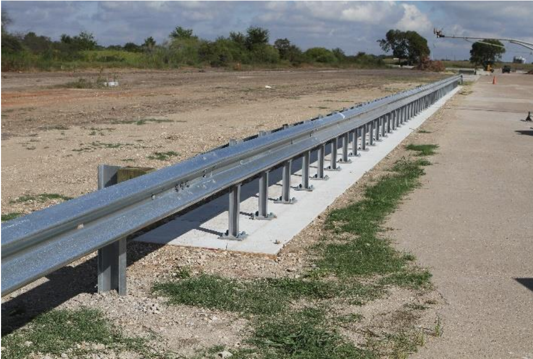
Figure 1. Surface-Mounted Median Guardrail.
