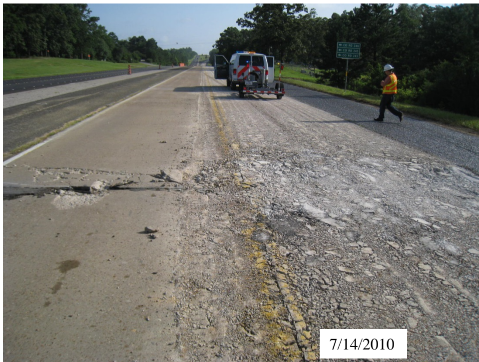
Figure 24. Rubblized (rubble) Concrete Conditions on One of the Worst Joints.
