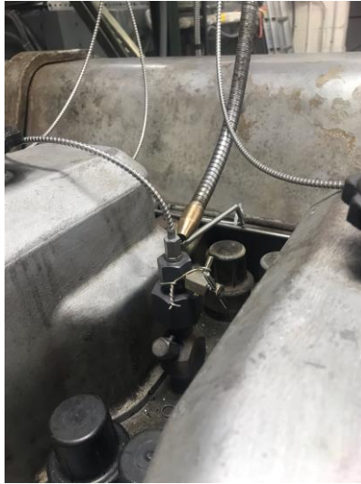
Figure 5: In cylinder pressure transducer attached to blow down petcock.
