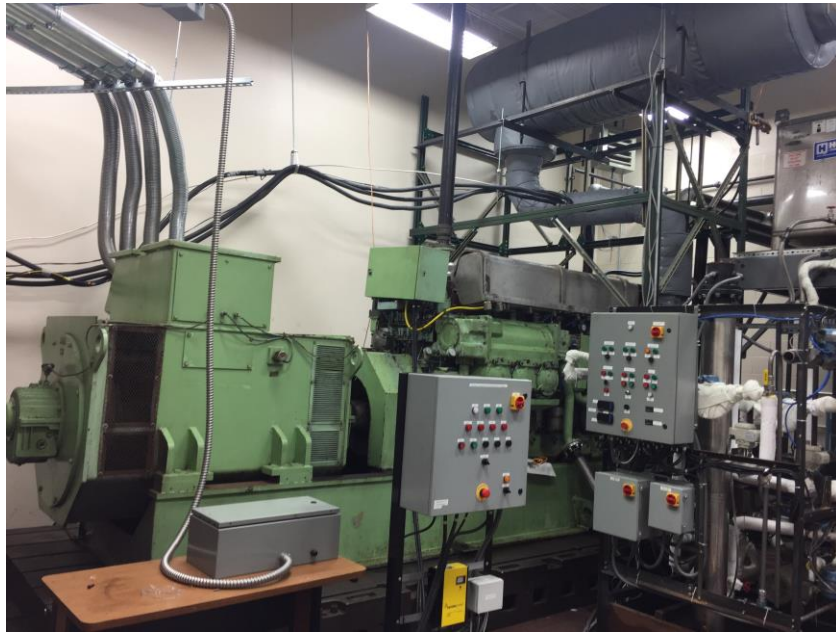
Figure 2: Medium Speed Engine Lab Completed
