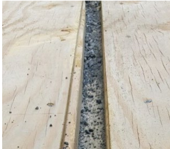
Figure 5. Simulated bridge expansion joint for on-site testing
