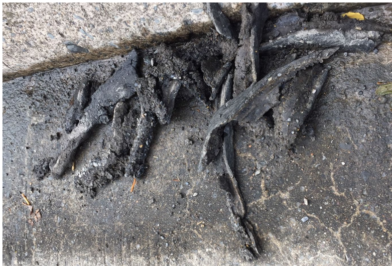
Figure 12. Pieces of sealer that were manually removed from bridge joint
