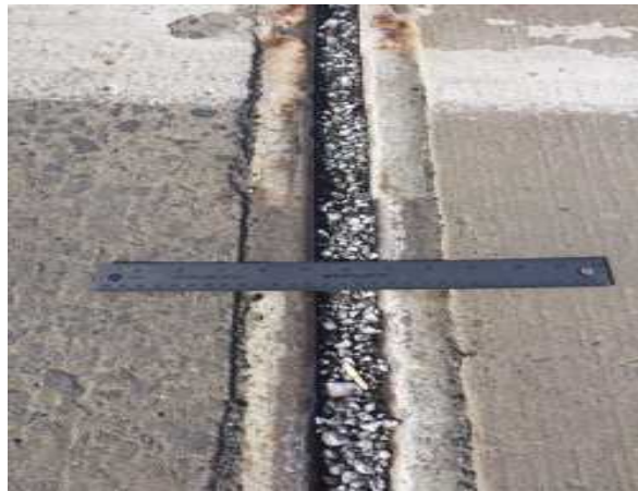
Figure 2. Sealed bridge expansion joint with contamination
