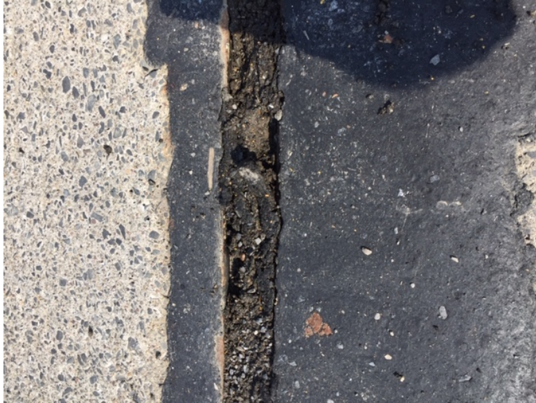
Figure 11. Bridge joint contaminated with sealer and debris
