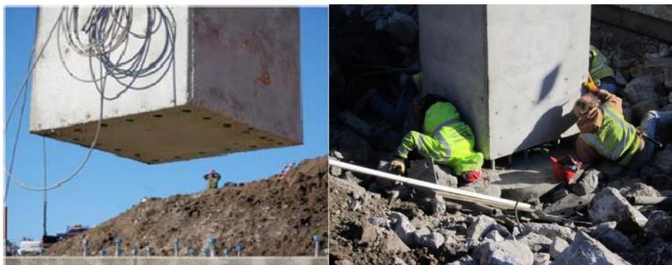
Figure 2-53: Precast column installation using grouted splice couplers in Keg Creek Bridge (Littleton 2013)
