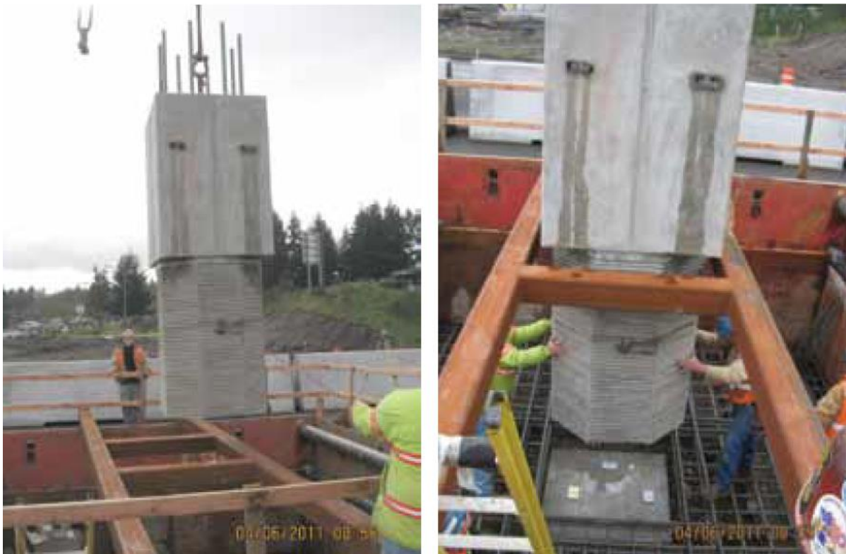
Figure 2-76: Socket connection between precast column and footing in US 12 bridge (Khalegi et al. 2012)
