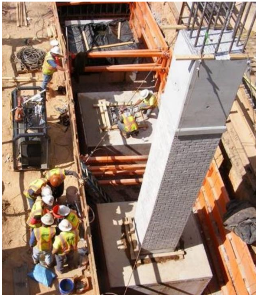
Figure 2-39: Erection of the precast column in Moore's Mill Road Bridge (City of Auburn 2019)
