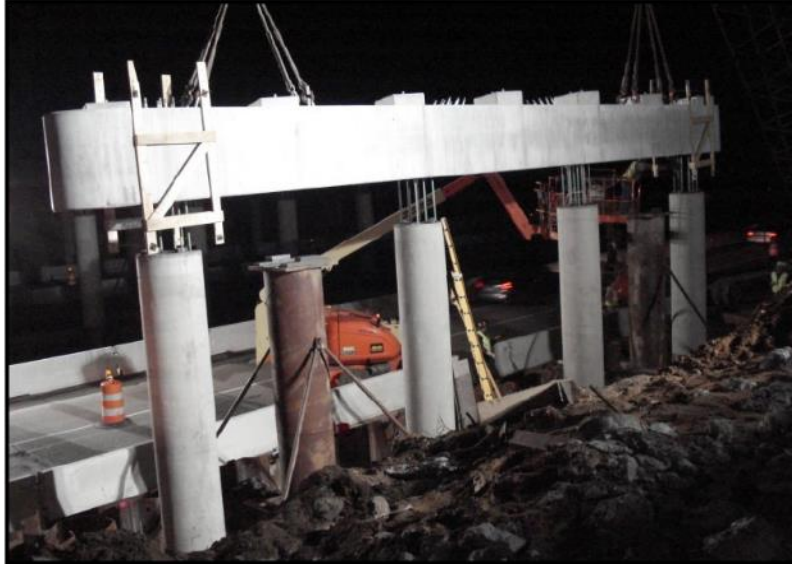
Figure 2-58: Precast bent cap being erected in Parkview Avenue Bridge (Attanyake et al. 2012)
