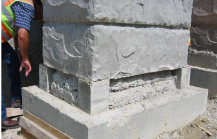
Figure 2-70: Base of precast column shell after core concrete filling, LP 340 over IH 35 (Wolf 2005)
