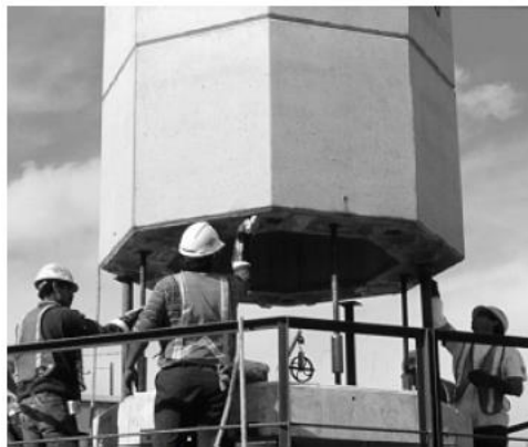
(c) PT bars coupled, placement of subsequent segments with epoxy applied to adjoining segment faces
