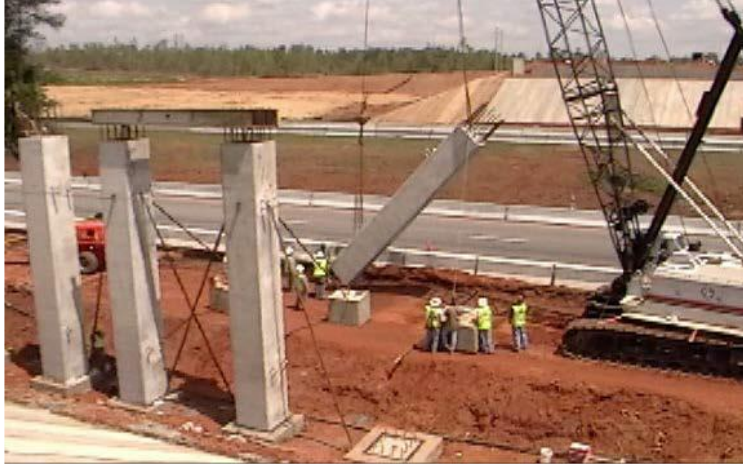
Figure 2-49: Erection of precast columns in the IH-85 Interchange project (Mallela et al. 2013)
