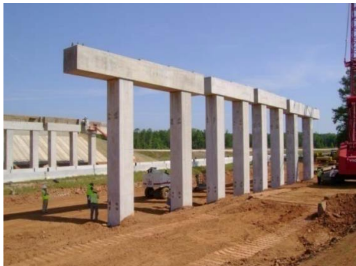
Figure 2-50: Precast columns and pier caps in the IH-85 Interchange project (Mallela et al. 2013)
