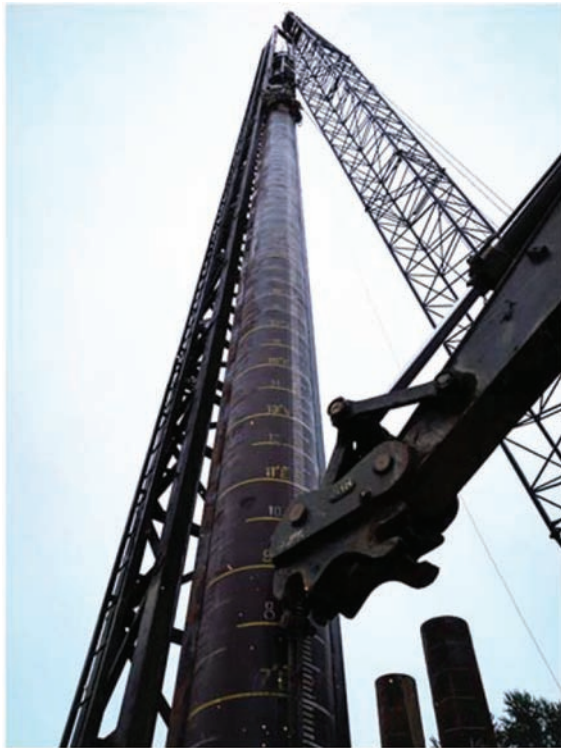
Figure 4.1 CEP being driven into the ground with a single-impact diesel hammer positioned on the top and a guiding frame around the CEP to ensure verticality during driving. (Modified after Ganju et al., 2018.)
