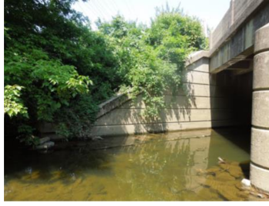
Photo 2 Span 1 Looking Down Stream Formation of Scour Hole
