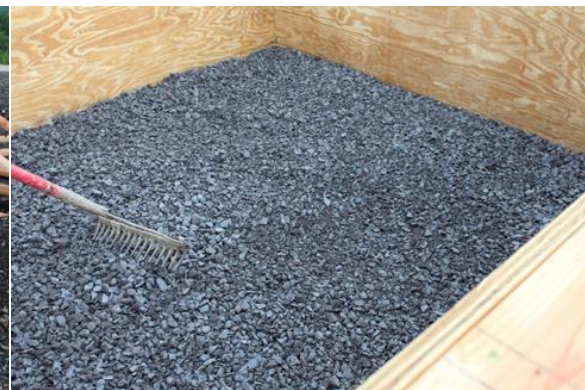
Photo 6 Six-inch Number 57 Type A Aggregates Spread on Top of the Geotextile Class 4, Type A
