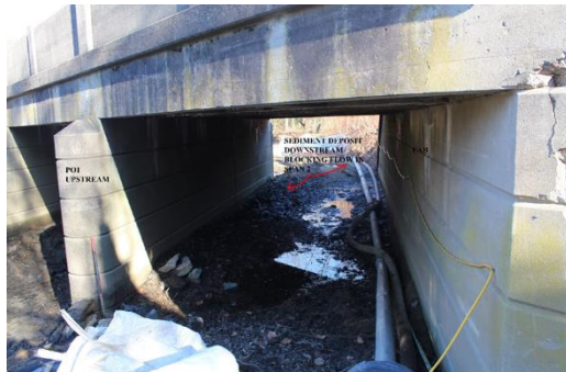
Photo 20 Pump discharge pipe in Span 2
