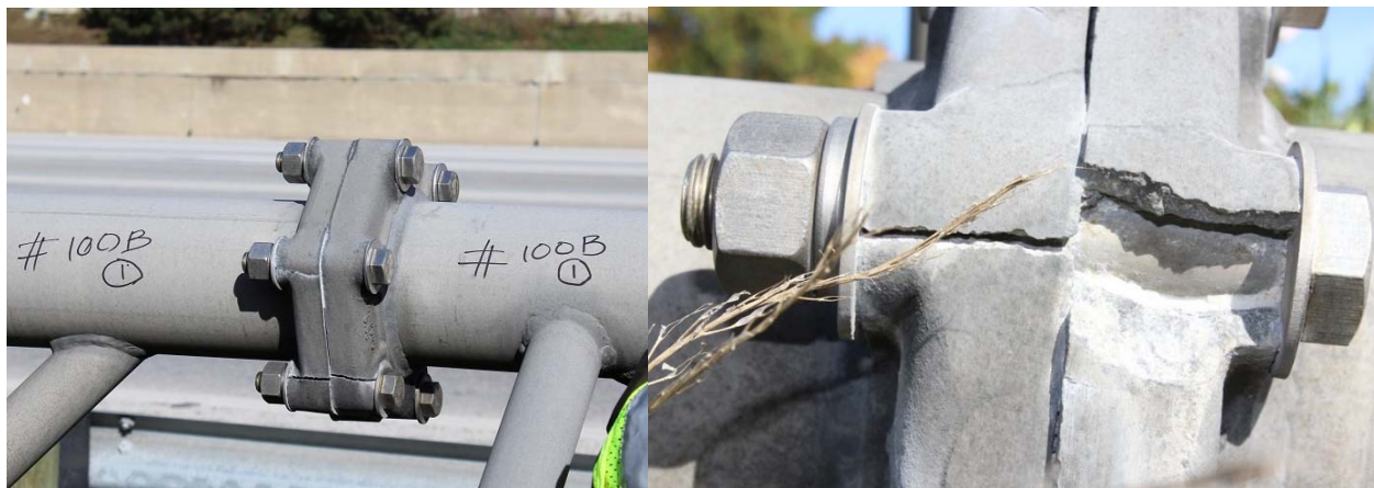
Figure 1: Typical Cracking (left) and Severe Cracking (right)
