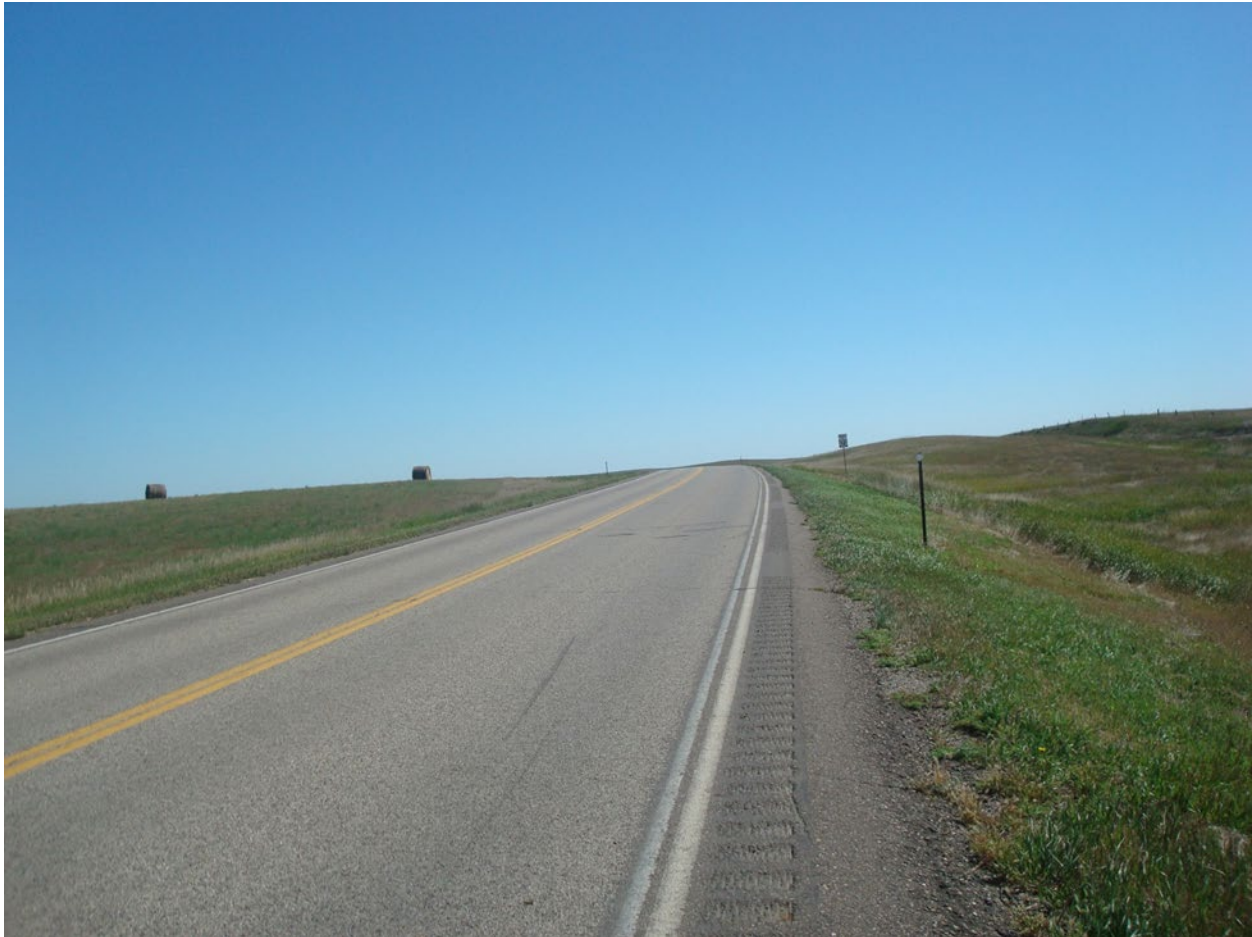
Figure 5.10 Reverse Superelevation at Curve on US 12 (MP 116.3)
