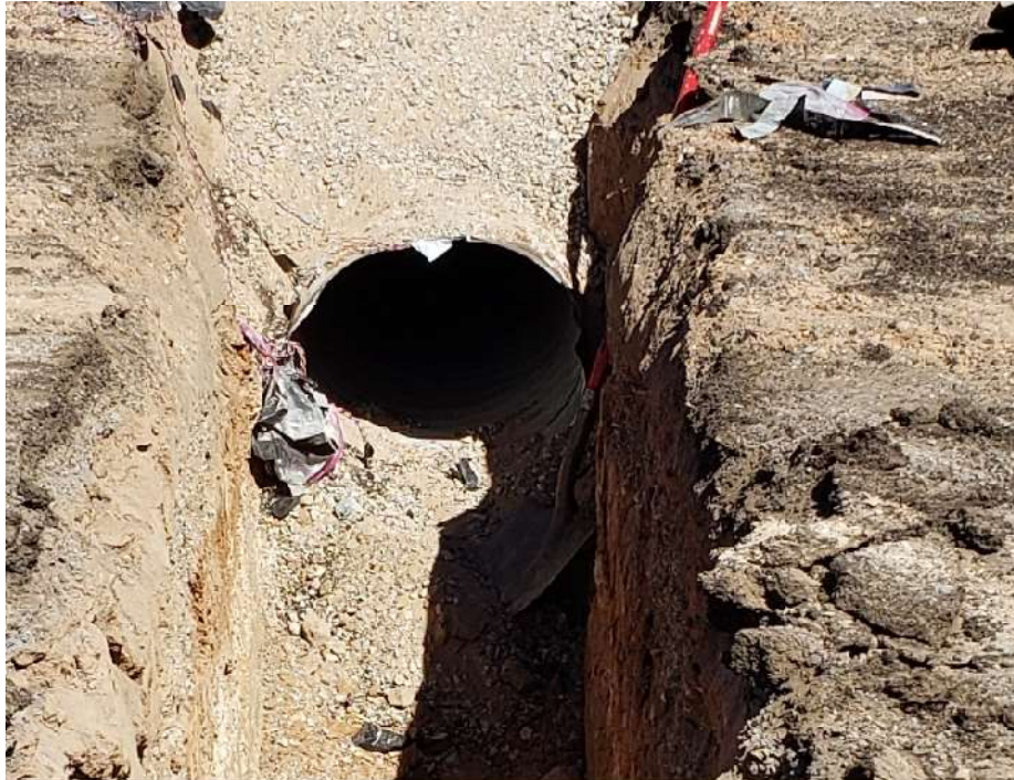
FIGURE 13 Buried corroded metal pipe
