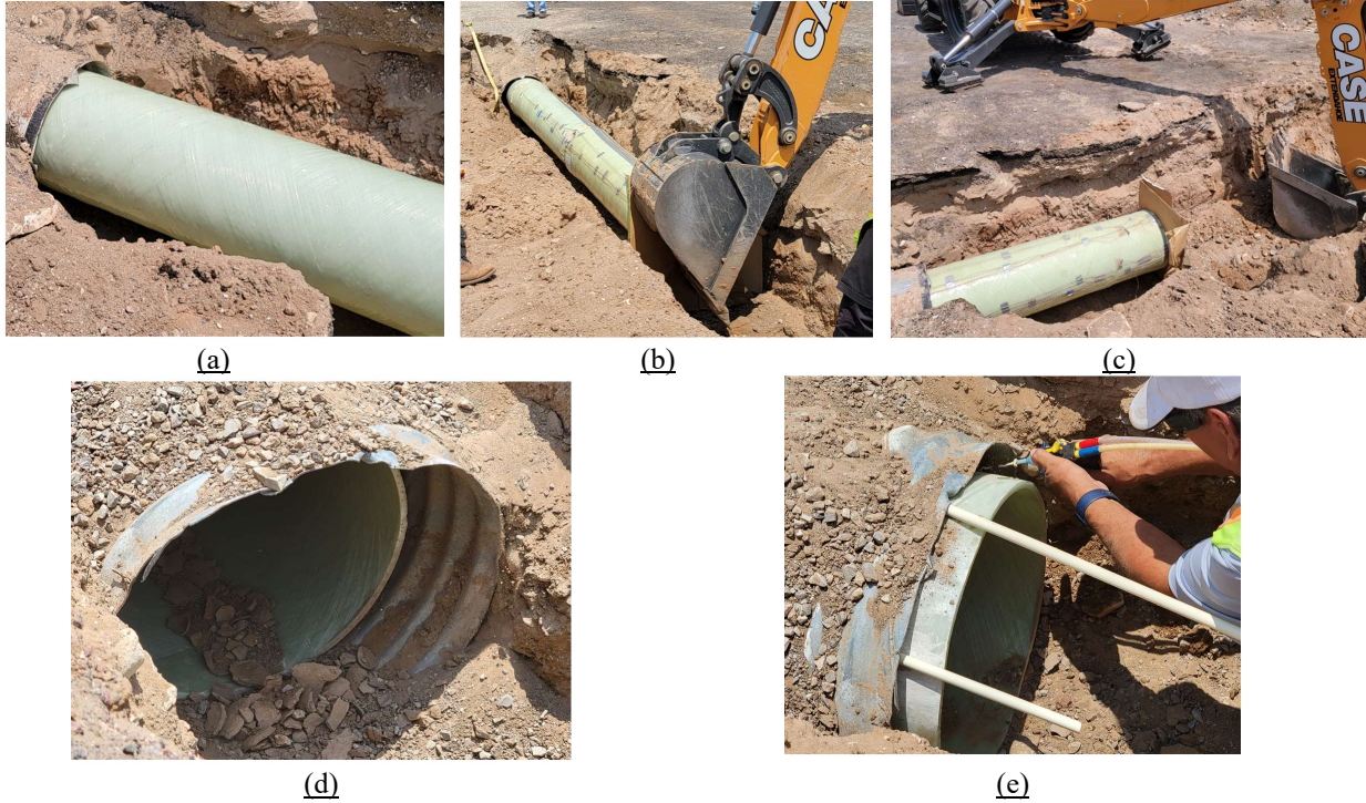
FIGURE 21 (a)-(c) Slip-Lining Process driving the GFRP pipe inside the corrugated metal culvert. (d)-(e) GFRP pipe completely slid inside the corrugated metal culvert and application of the closure foam prior to grouting of the annular space.
