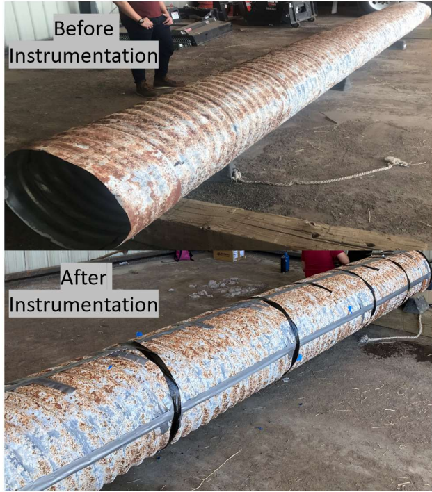
FIGURE 11 Corroded metal pipe before and after instrumentation
