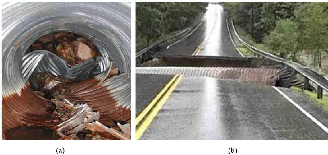
FIGURE 2 Failure of corroded metal culverts [2].
