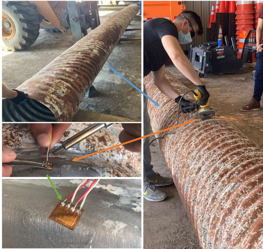
FIGURE 12 Instrumentation of corroded metal pipe
