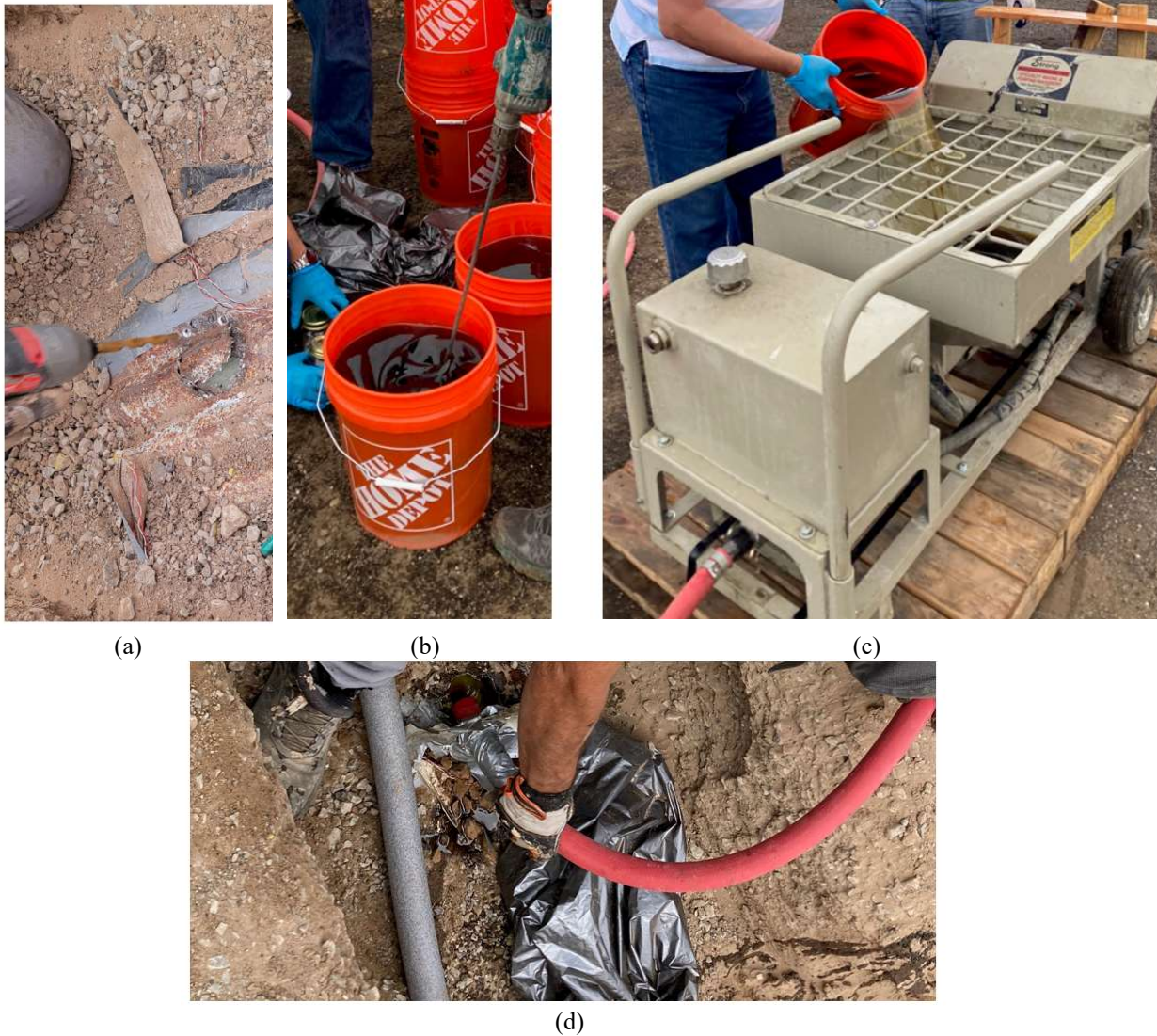
FIGURE 23 Mixing and pumping polymer in the annular space using an opening at the middle of the span. (a) perforation to inject polymer. (b) polymer mixing. (c) polymer pumping. (d) polymer injection.
