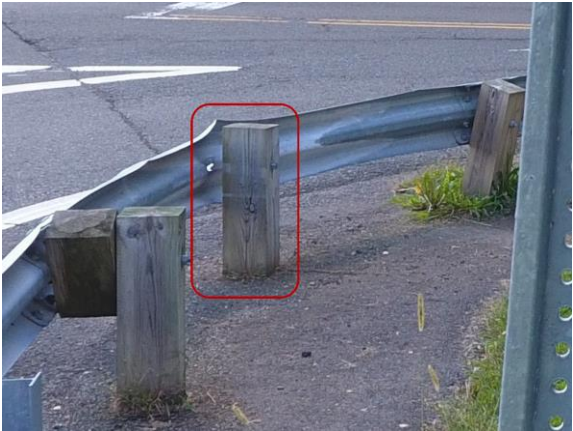
Figure 17: Guiderail Missing Connection
