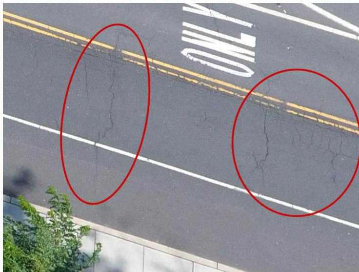
Figure 14: Asphalt Cracking Cont.
