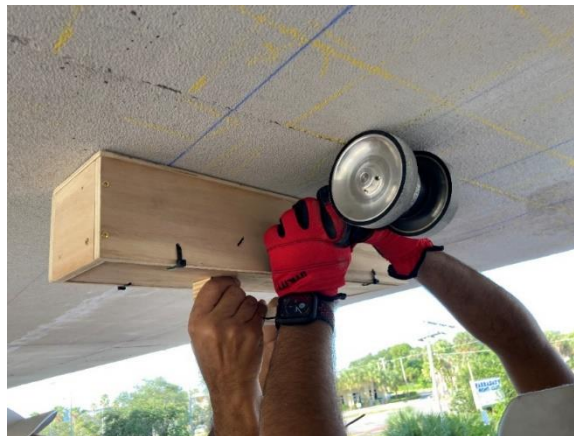
Figure B-37: Obtaining MFL signal from the bottom side.
