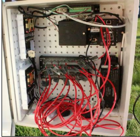
Figure 2.5: CR1000 Data-Logger (top-right) in weather-proof box. Decagon Devices Em50 Data Loggers (left side)
