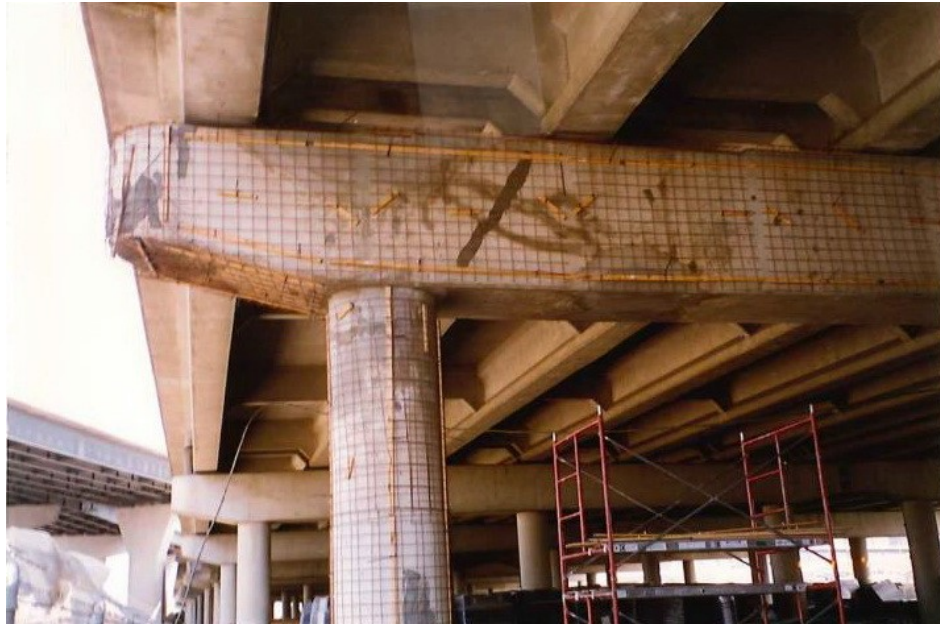
Figure 2.13 Pier 37WB - ECE installation in progress, prior to application of cellulose fiber
