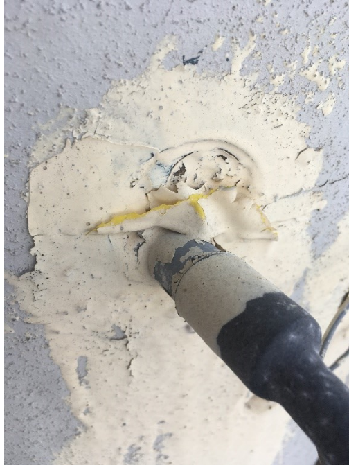
Figure 4.8 Pier 37WB [ECE] - Sealant at perimeter of instrument penetration through FRP (2018)
