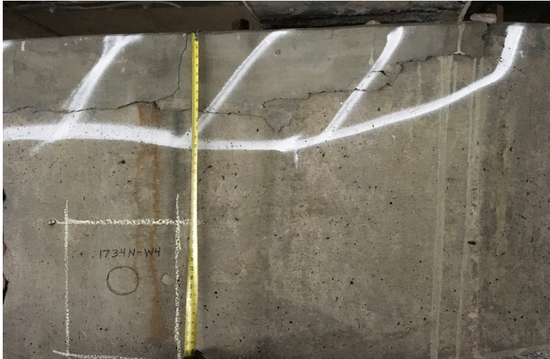
Figure 3.1 Pier 34WB - Example of distress identified on the west face of the pier cap
