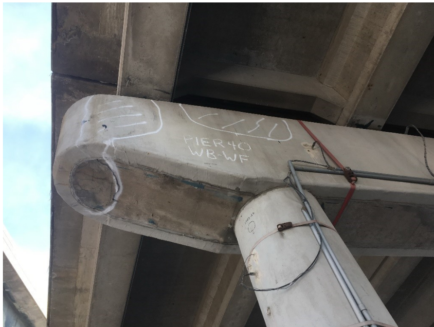
Figure 4.7 Pier 40WB [Non-ECE] - No FRP coverage of bottom pier cap surface (2018)
