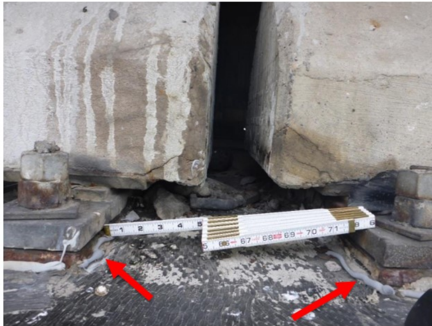
Figure 4.9 Pier 34WB [ECE] - Sealant at precast bearings on top of pier cap (2018)
