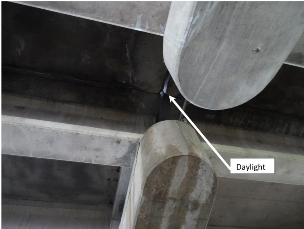
Figure 3.22 Pier 34WB - Daylight at deck joint and moisture staining below on end of pier cap.
