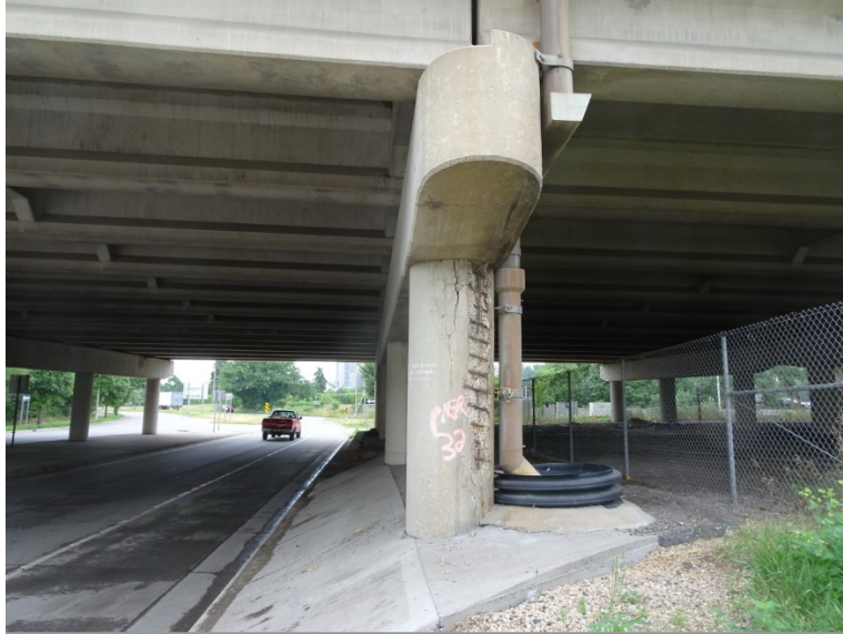
Figure 1.1 Typical corrosion damage in concrete bridge substructures
