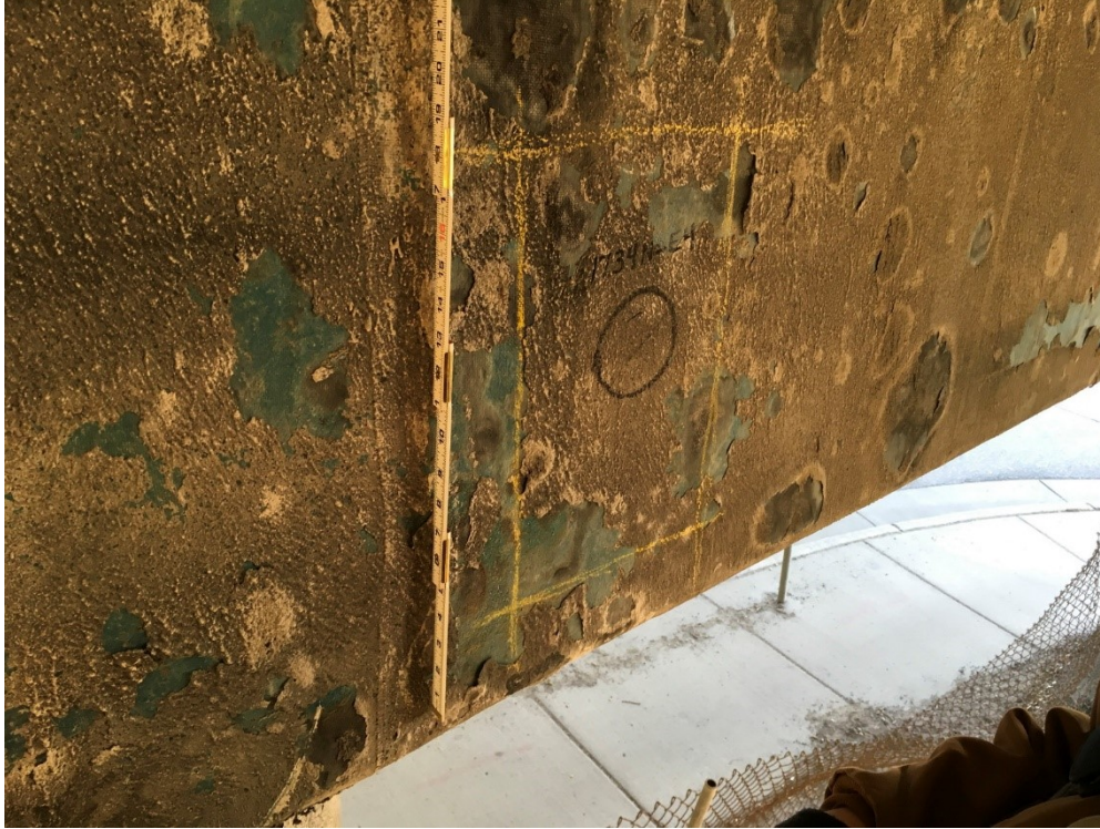
Figure 3.24 Pier 34EB - Fire damage to FRP applied on east face
