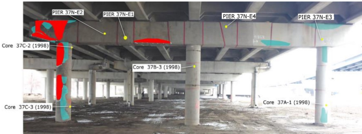
Figure 3.30 Pier 37WB [ECE] - East face - Delaminations in 2018 (red) and 1998 repair areas (blue)
