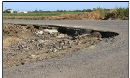
Figure 3.6: Road damage caused by high intensity rainfall.
