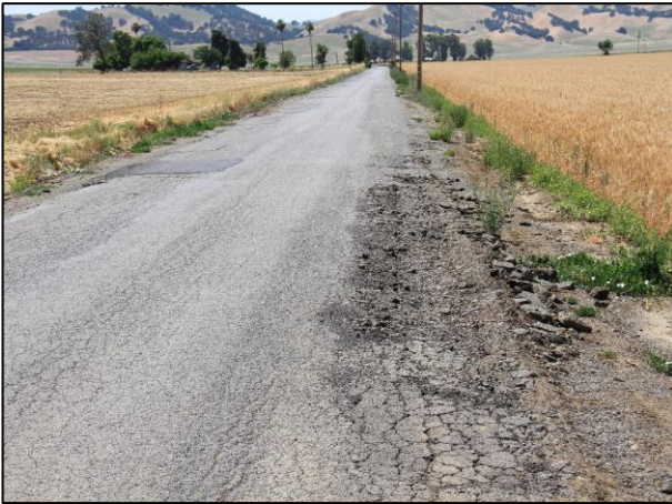
Before (Severely Distressed Paved Road)
