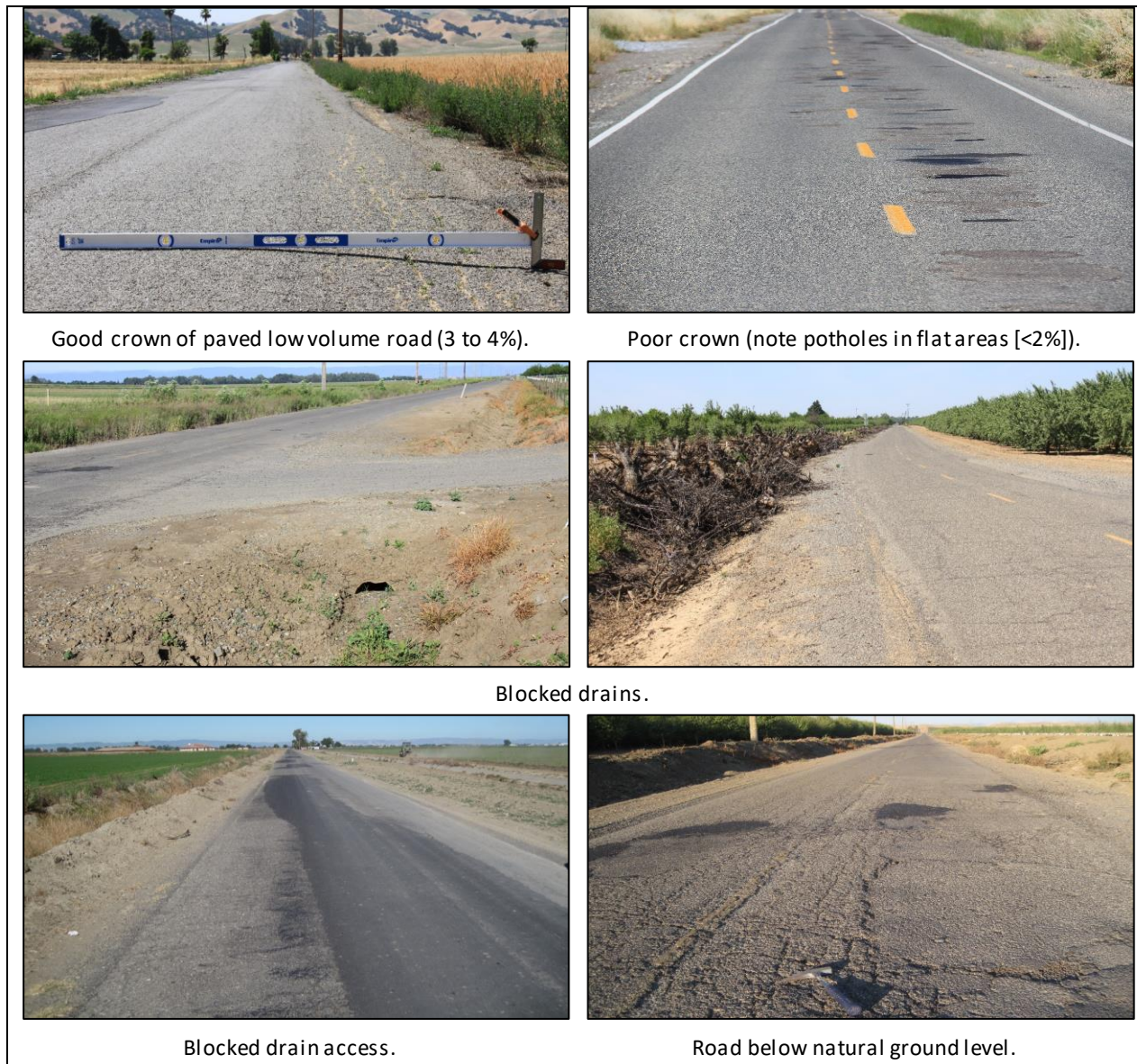
Figure 3.14: Examples of drainage problems.
