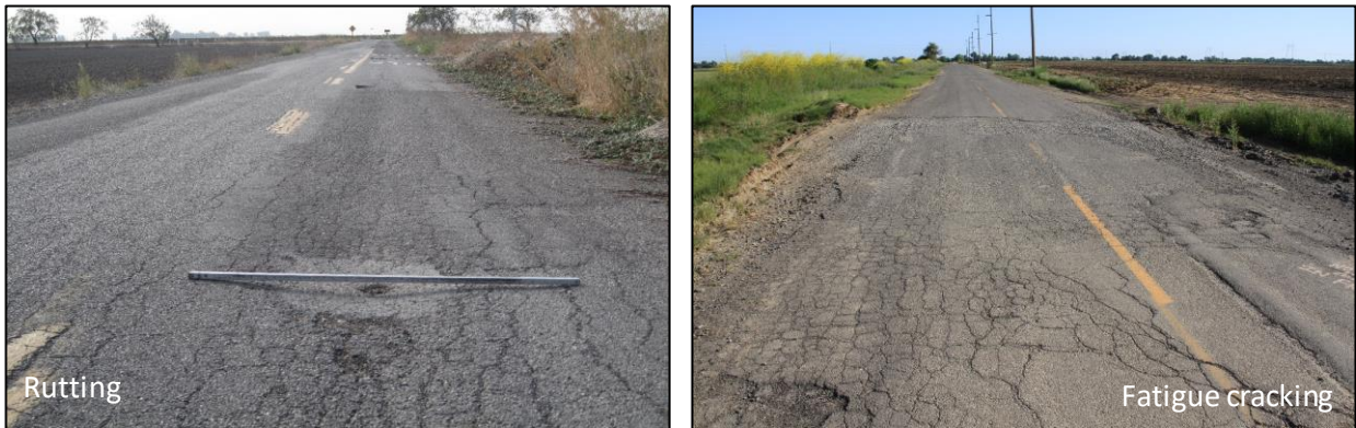
Figure 3.11: Examples of structural-related distresses.
