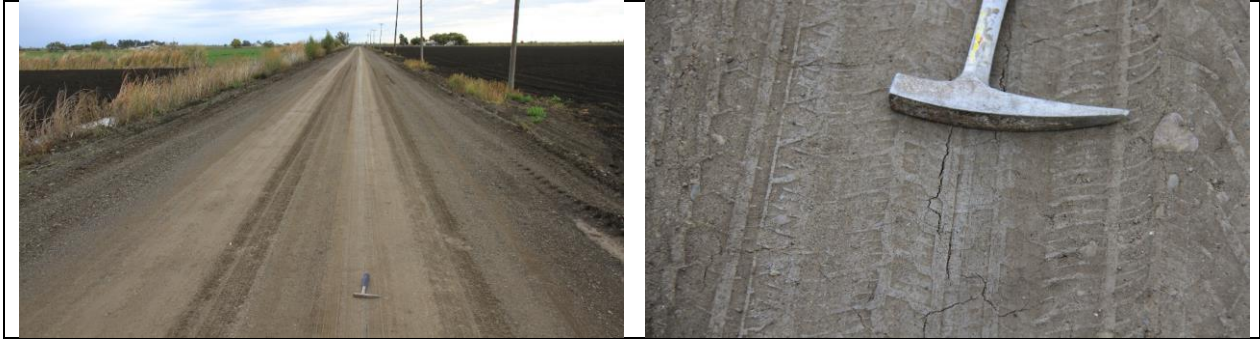
Figure 5.5: Excess fines resulting from exceeding the design depth during mixing.
