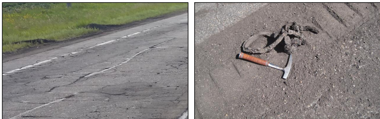
Figure 3.16: Example of cracked sealed road and sealant requiring manual removal during recycling.
