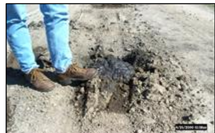
Figure 3.7: Road damage caused by frost boils.
