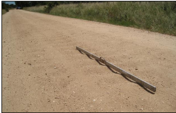
Figure 5.6: Washboarding resulting from not meeting the design mixing depth.
