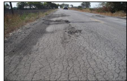
Figure 1.1 Distressed paved road.
