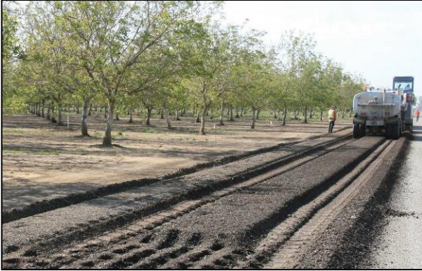
Figure 5.9: Differential compaction in recycling train wheelpaths.
