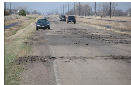
Figure 1.3: Safety concerns on distressed paved road.
