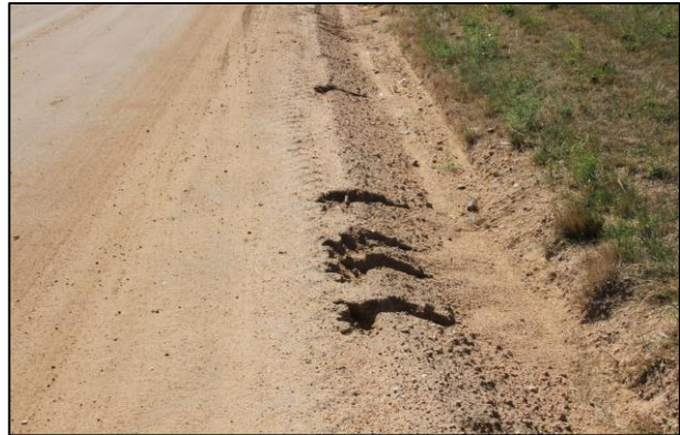
Figure 5.15: Windrows blocking water flow from the road.
