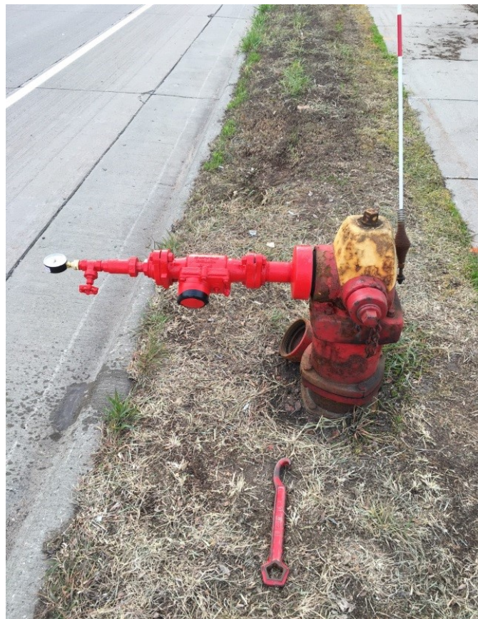
Figure 4.7 Hydrant connection with backflow prevention, meter, and wrench.
