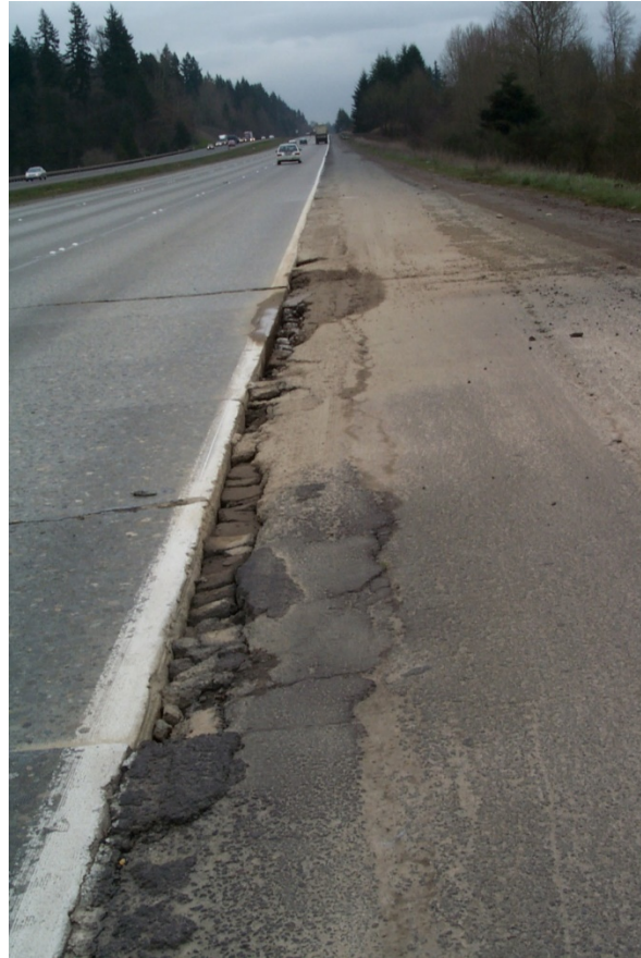
Figure 1.1 Damage caused by water pumping at the inner edge of the road shoulder
