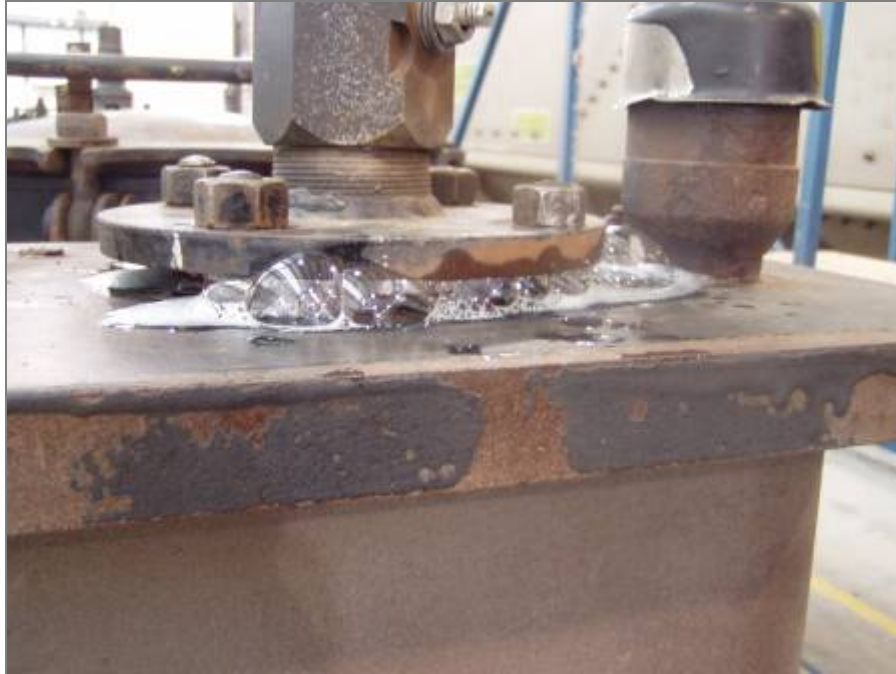
Figure 50. Leak at an Inspection Port
