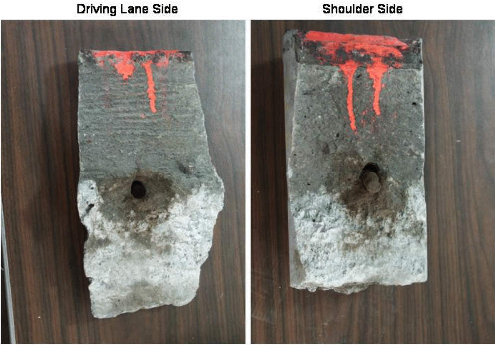
Figure 3. Shoulder Joint, Eastbound Station 1687+22
