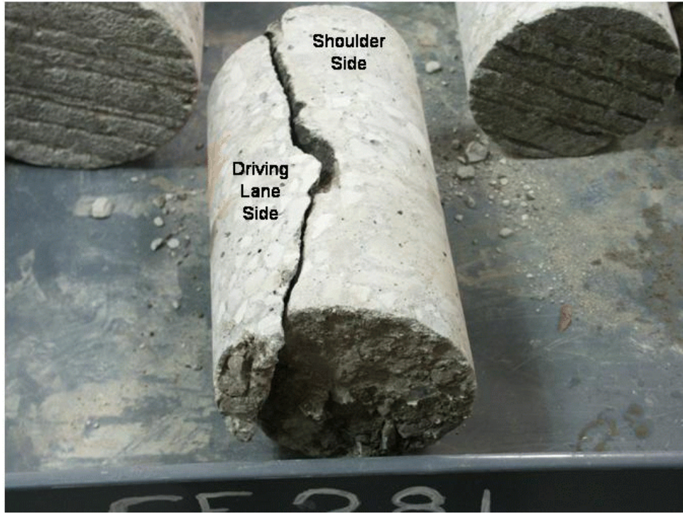
Figure 2. Shoulder Joint, Eastbound Station 1687+22
