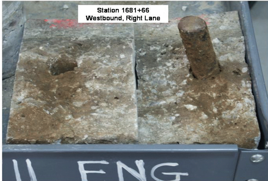
Figure 6. Transverse Joint Dowel Bar, Right Lane Westbound Station 1681+66
