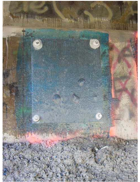
Figure 3.4: Patch with delaminations shown.
