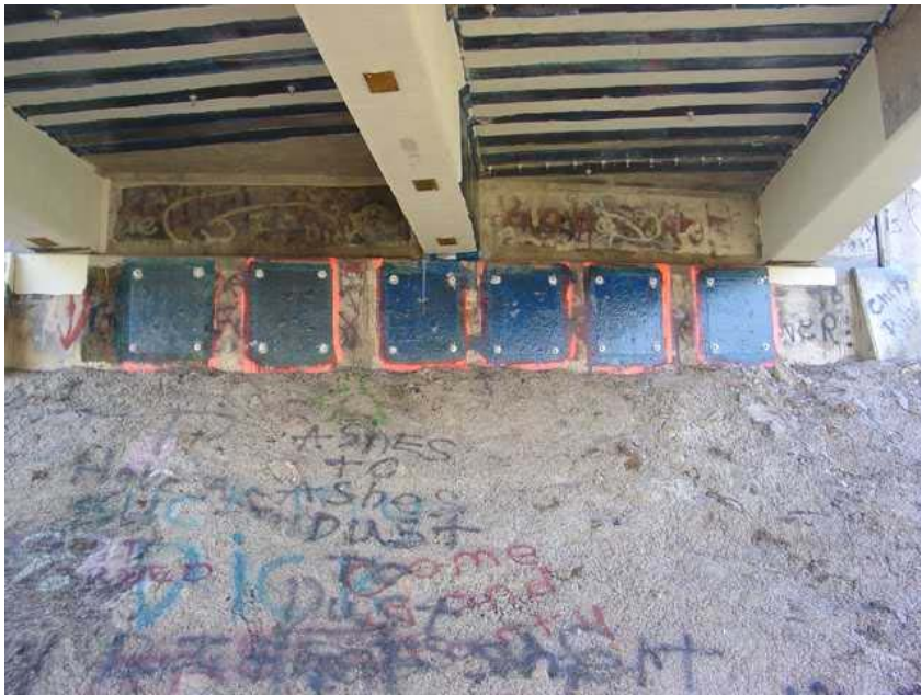
Figure 3.3: Panels for delamination on south abutment.
