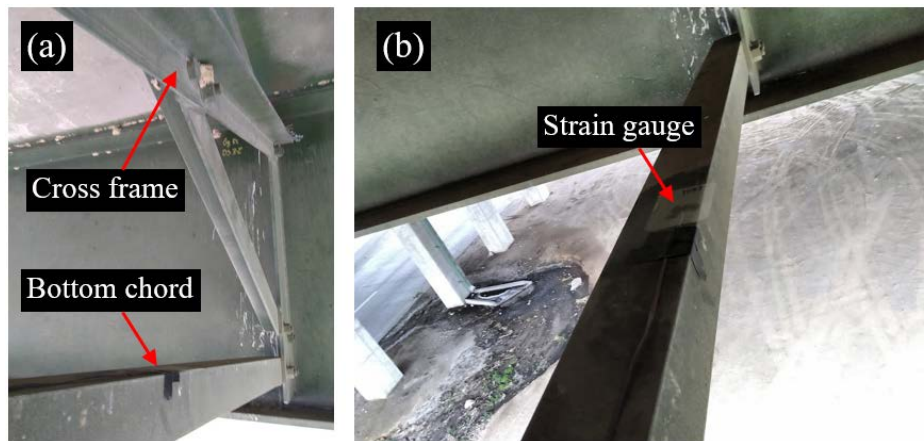
Figure 6.18: Strain Gauge Installation on the Cross Frame (a) Cross Frame Prior to Sensor Installation; (b) Strain Gauge Installation
