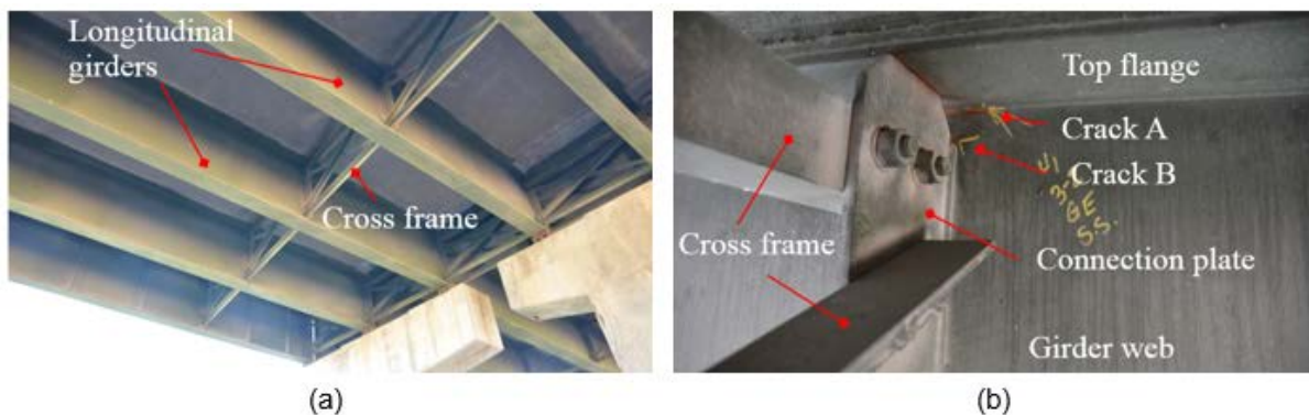
Figure 4.2: (a) A Typical Structural Layout of a Steel Girder Bridge in the Field; (b) Representative Distortion-Induced Fatigue Cracks at the Web-Gap Region
