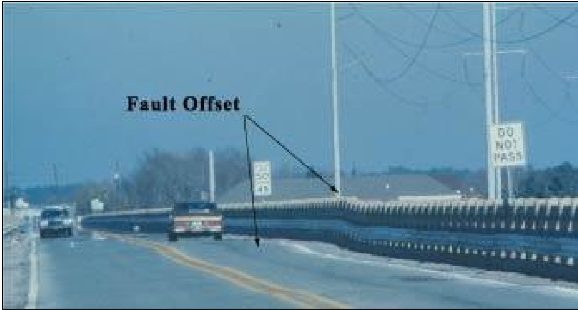
Figure 3. Photograph of fault induced offset in the Highway 11 Bridge that crosses Lake Pontchartrain (5).
