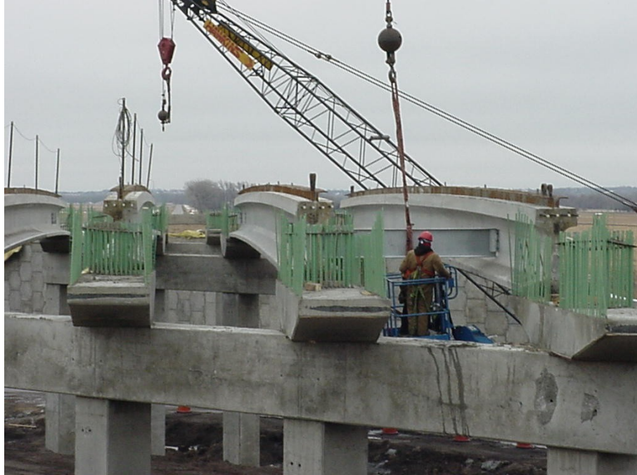
Figure 4.10 View of Precast Girders Placed over Pier Haunch along the Traffic Direction
