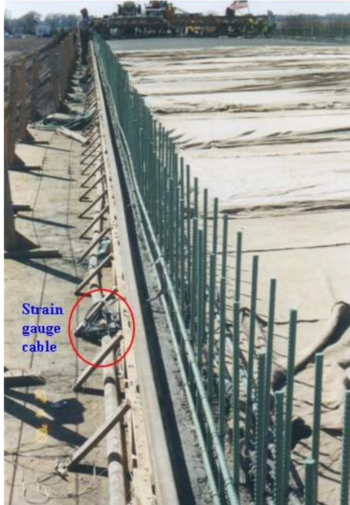
Figure 4.21 Strain Gauges in the Construction Field
