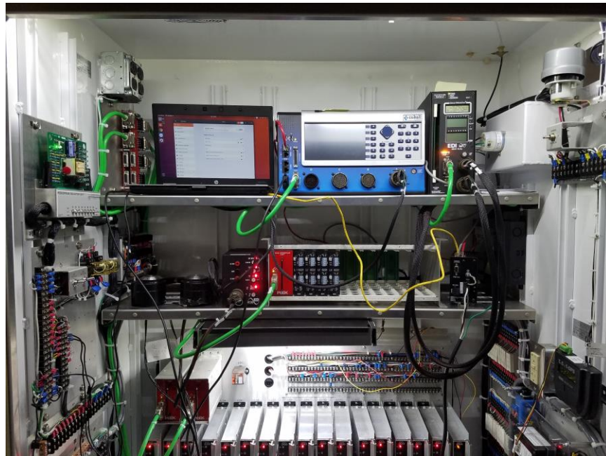
Figure 7.6 Inside of the traffic cabinet, including the controller, MMU, and switch
