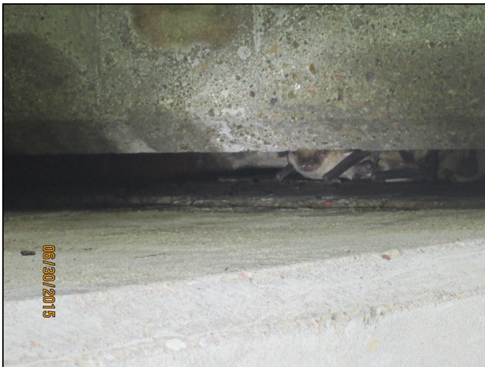
Photo 8: Bats in crevice of bridge. Orientation: South
