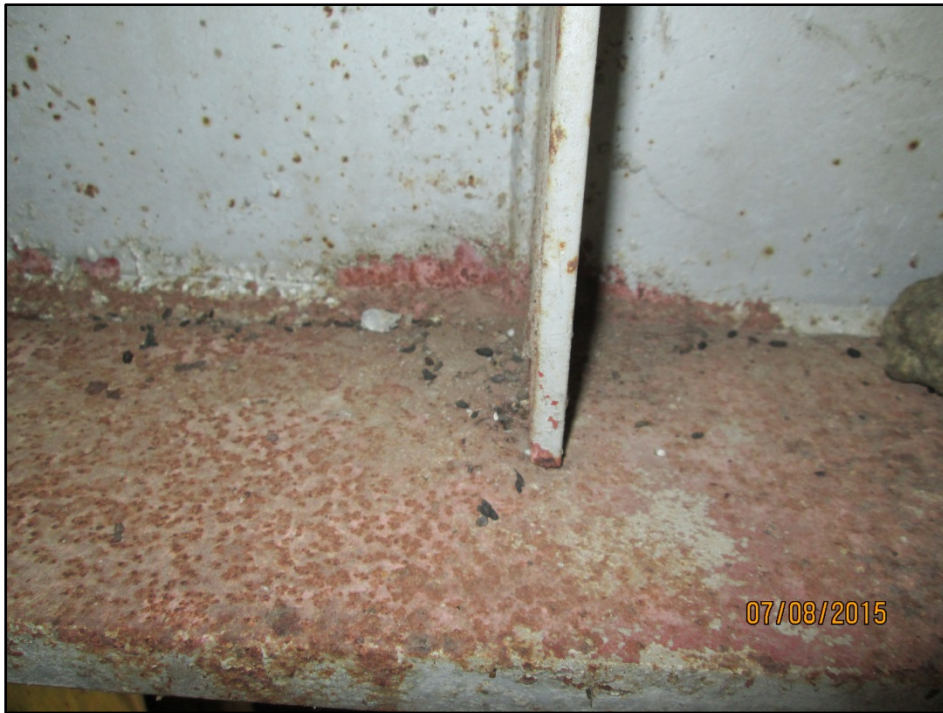
Photo 3: Bat guano near abutment Orientation: South
