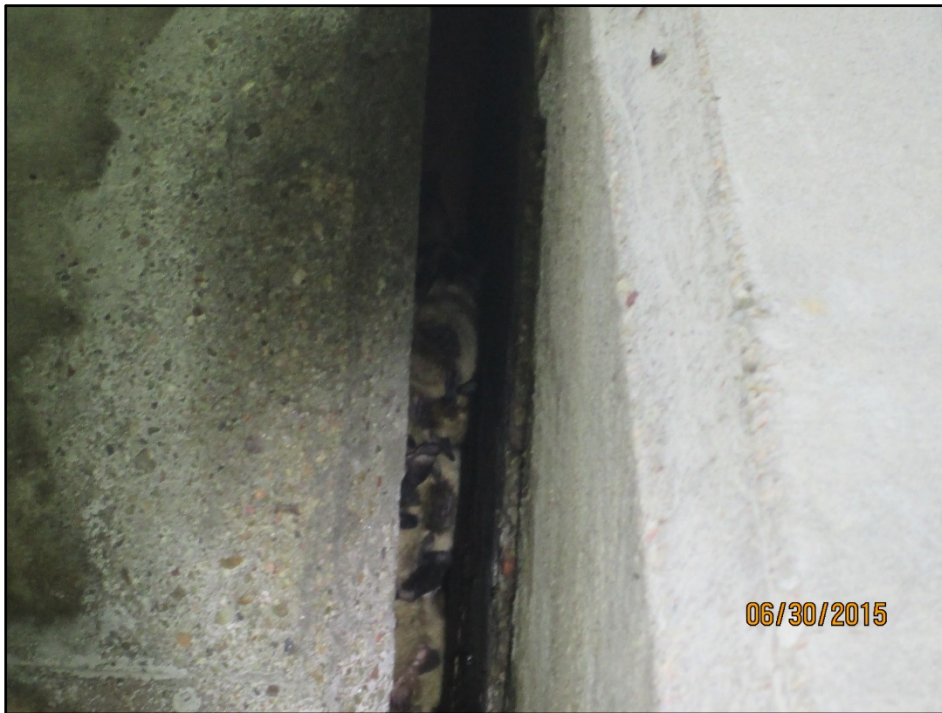
Photo 6: Bats in crevice of bridge. Orientation: South
