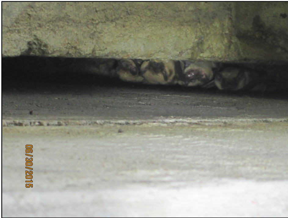
Photo 7: Bats in crevice of bridge. Orientation: South
