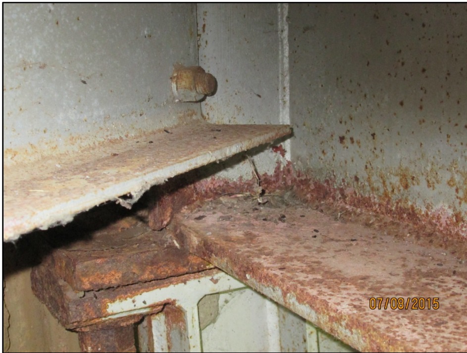
Photo 4: bat guano by abutment Orientation: East
