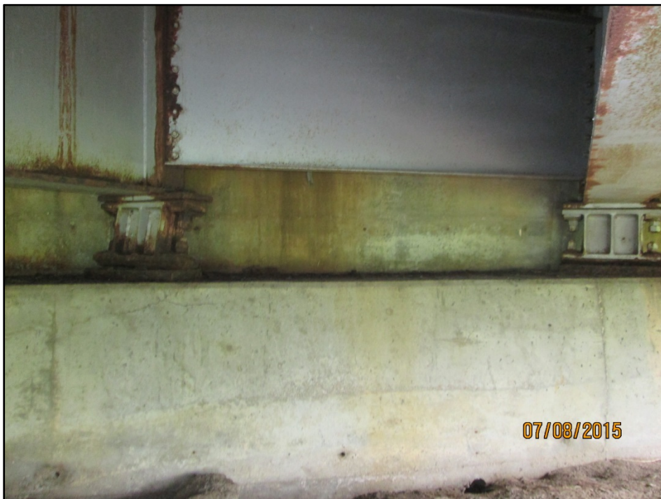
Photo 6: Abutment ledge where bat guano was found Orientation: East
