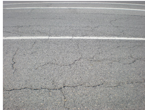
(b) Close-up of road showing cracks
