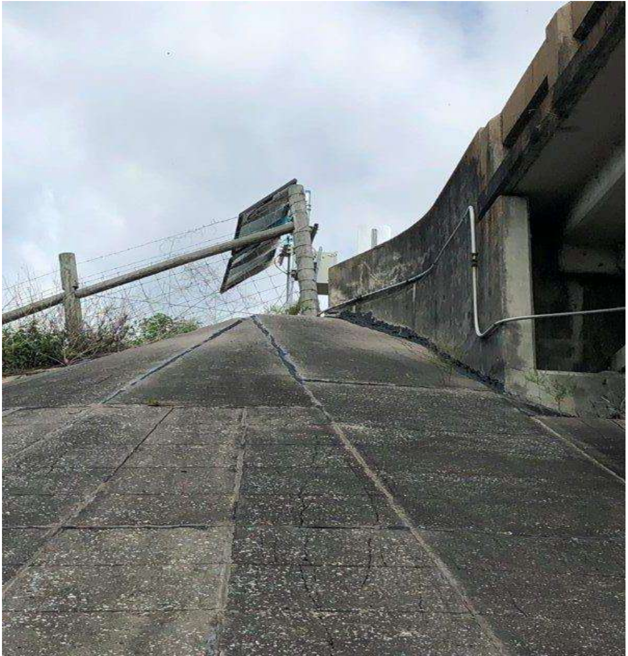
Figure 86: Solar Unit: Site 2
