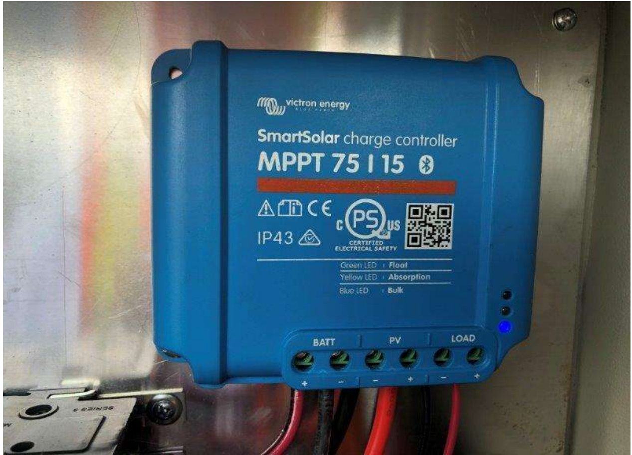
Figure 109: Site 2: Solar Controller
