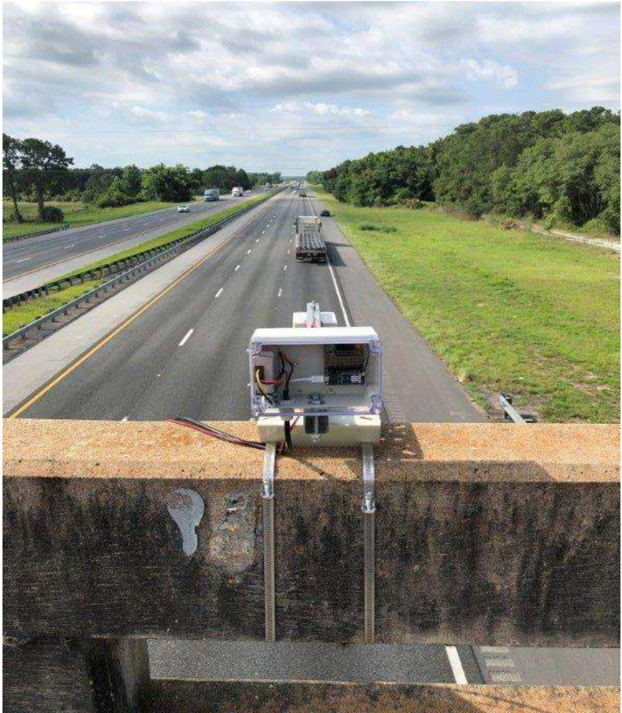
Figure 99: Site 2: Gateway Unit
