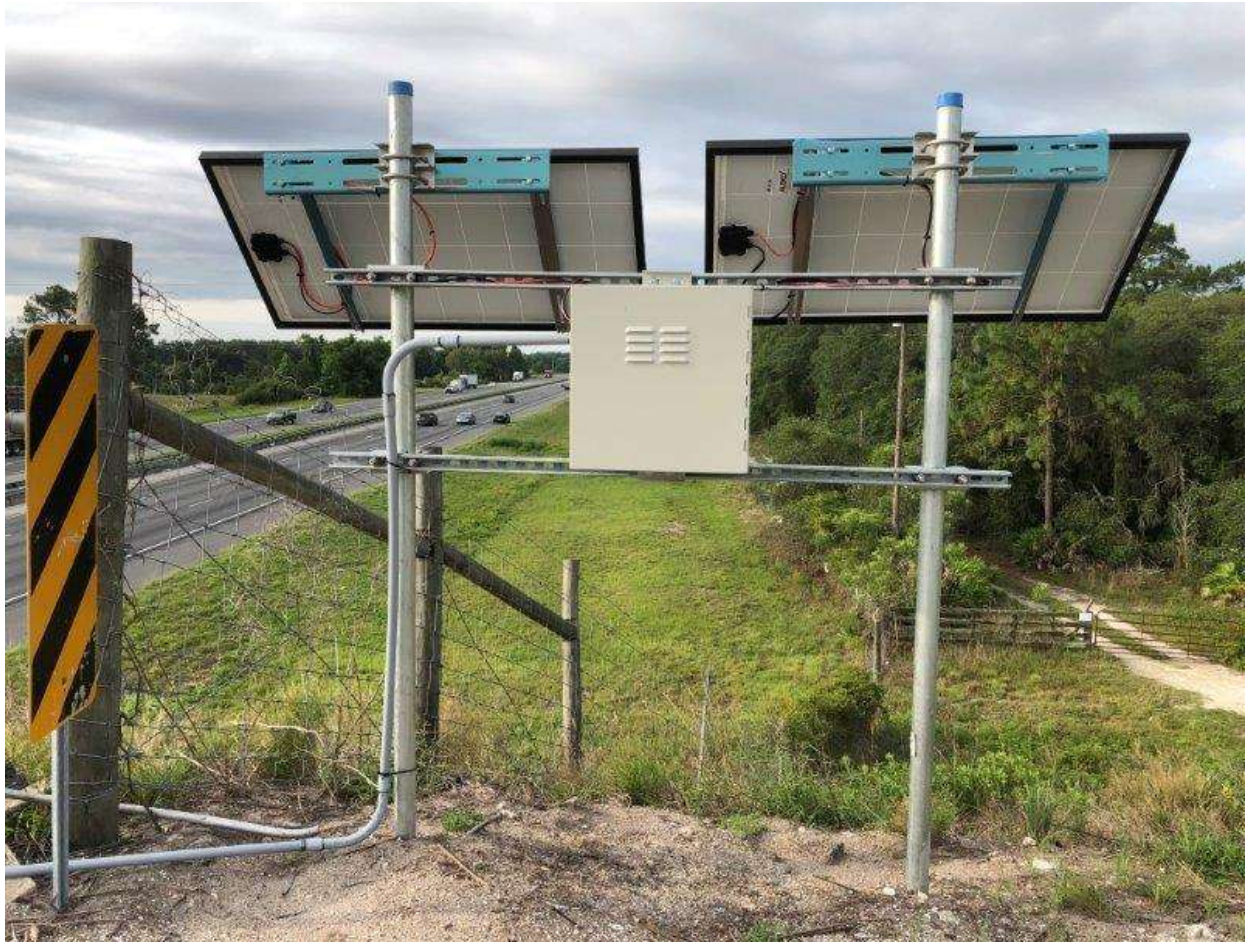
Figure 85: Solar Unit for Site 2 (6 Traffic Lanes)
