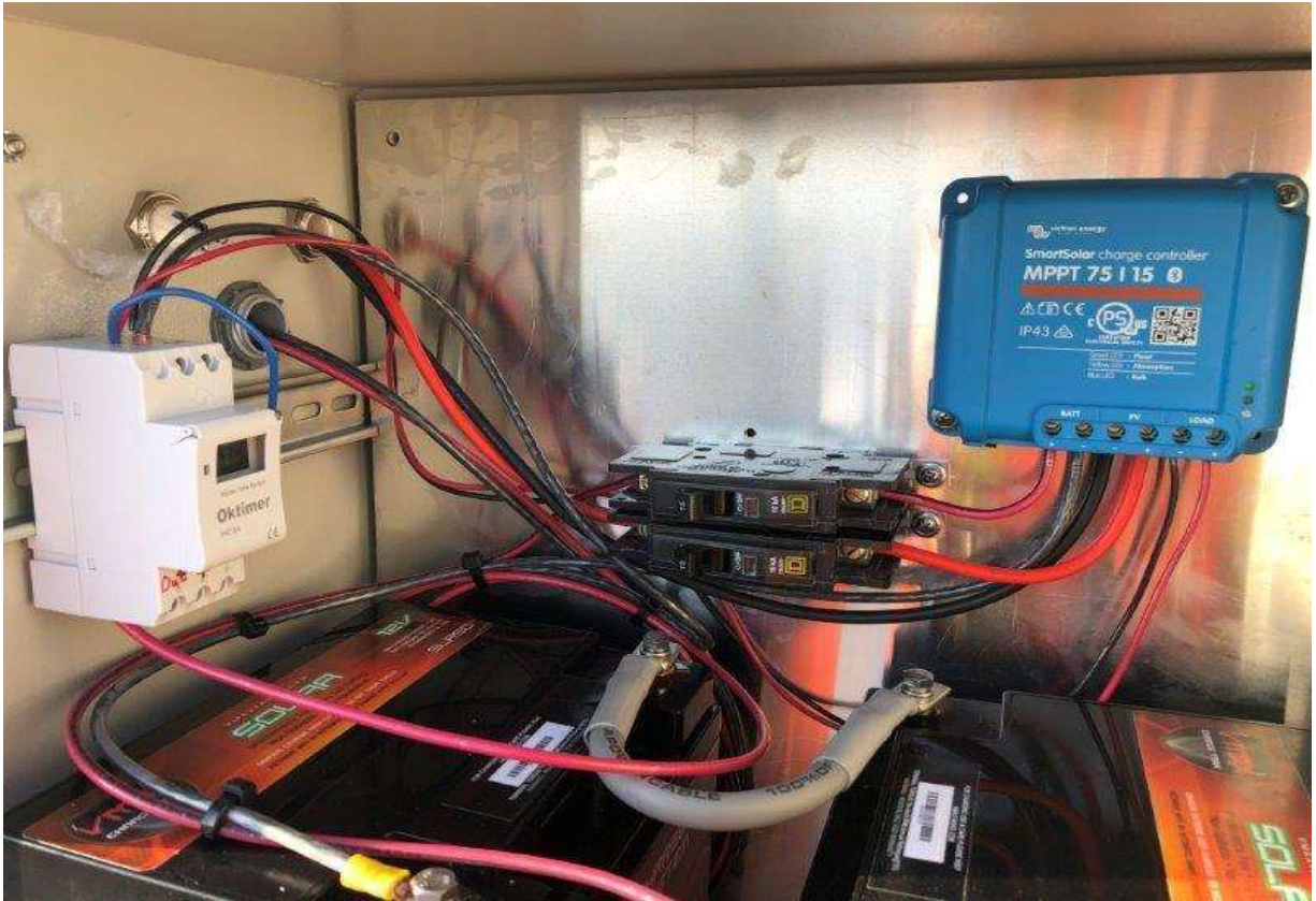
Figure 106: Solar Controller and Power Relay
