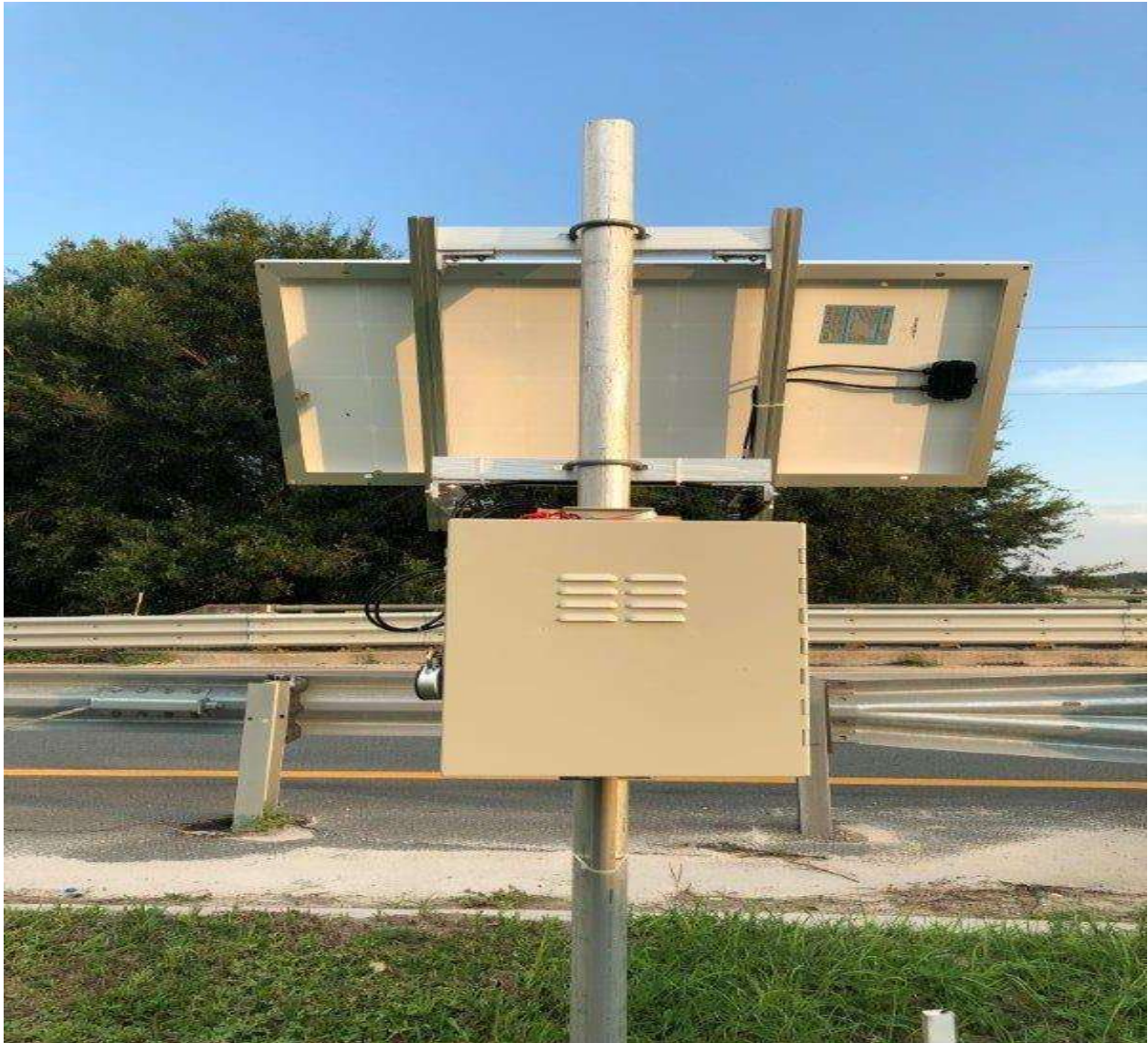
Figure 80: Solar Power Unit for Site 1 with Battery Box
