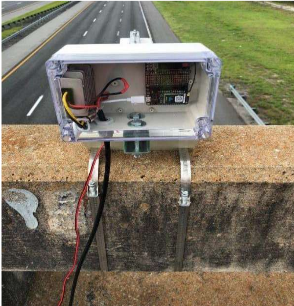
Figure 94: Site 2: Gateway Unit with Voltage Regulator
