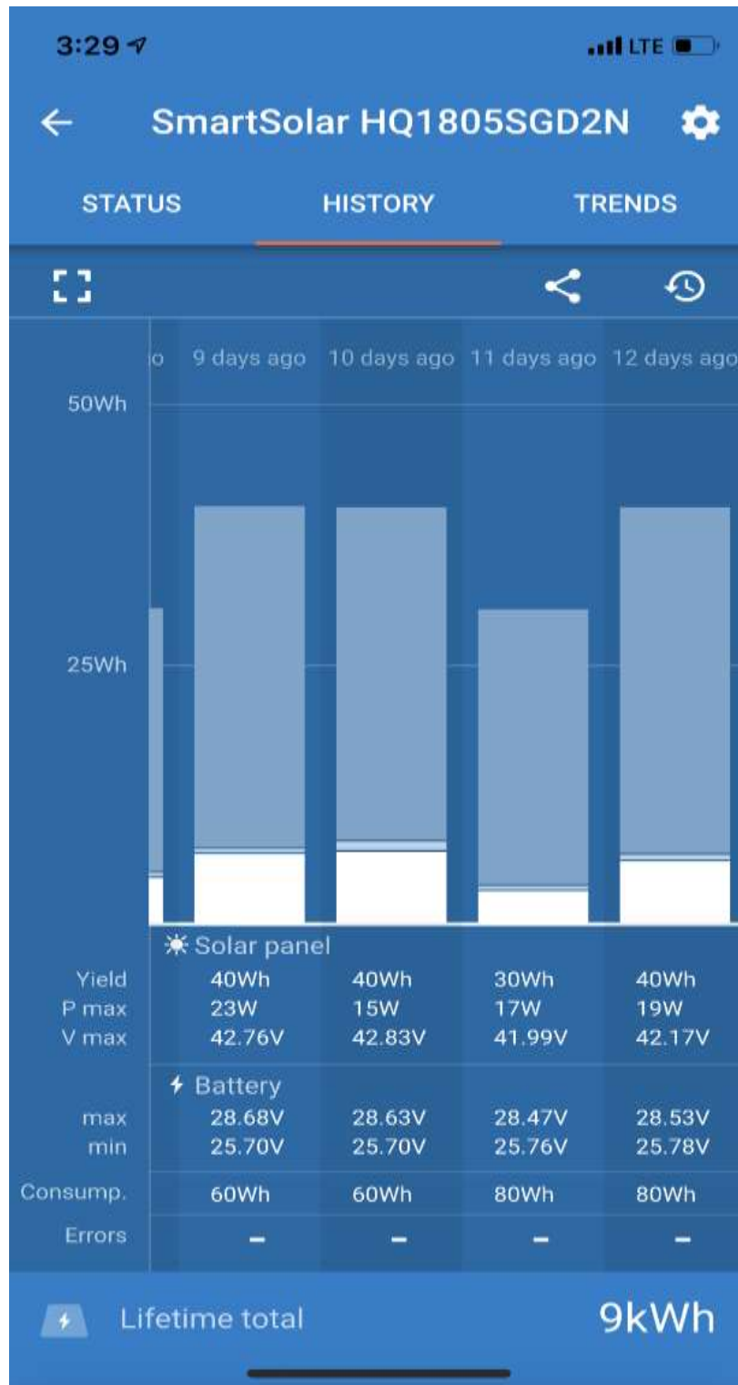
Figure 112: Solar Controller Display via Bluetooth
