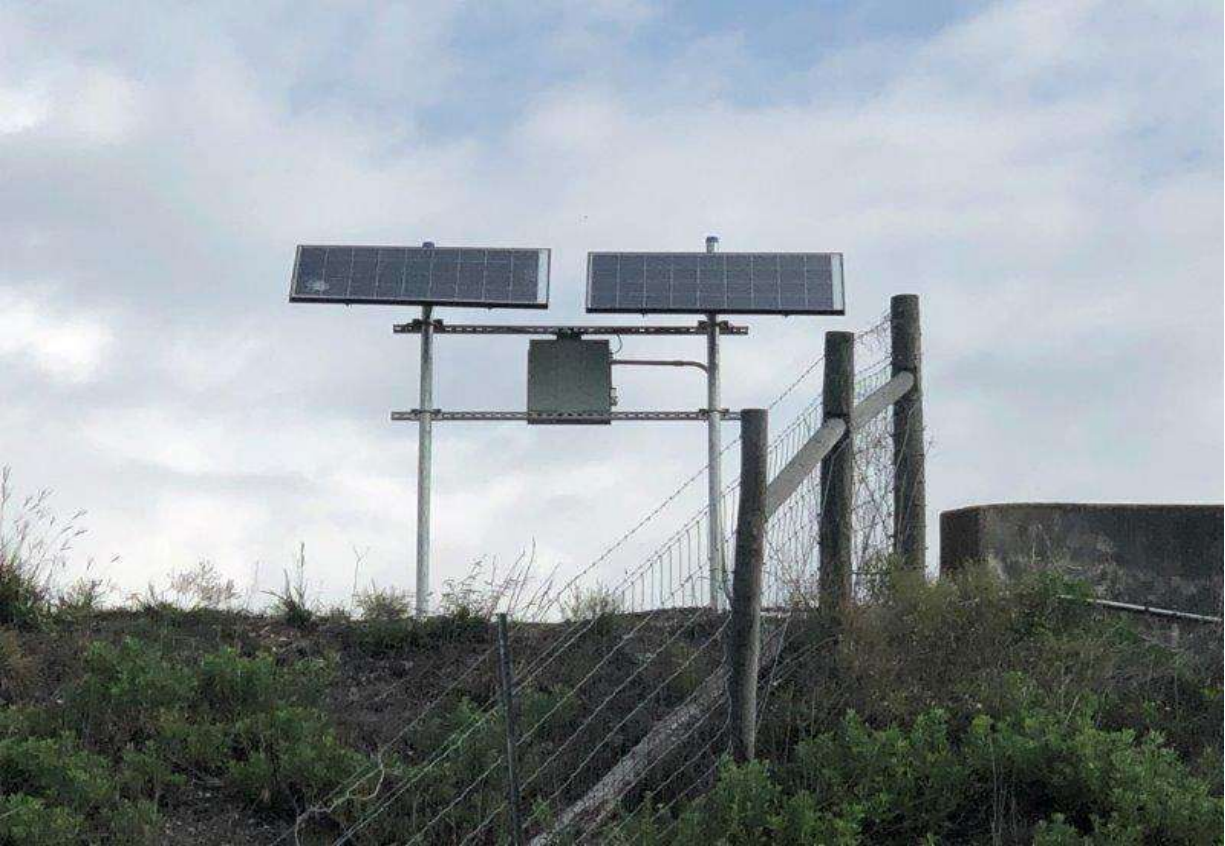
Figure 84: Solar Unit for Site 2 (24V)
