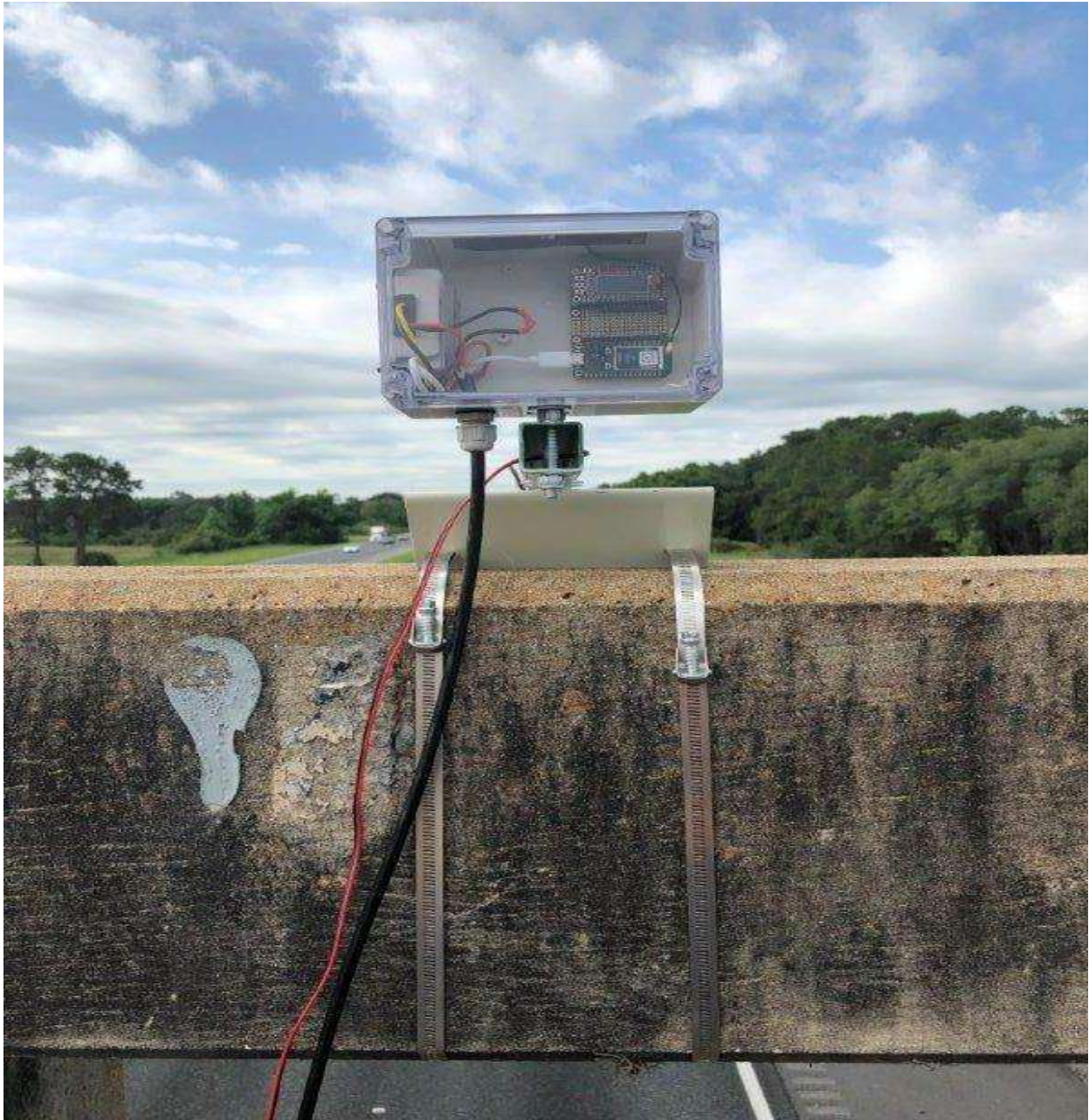
Figure 98: Site 2: Gateway Unit
