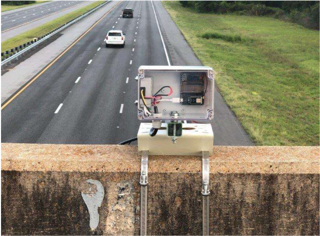
Figure 95: Site 2: Gateway Unit
