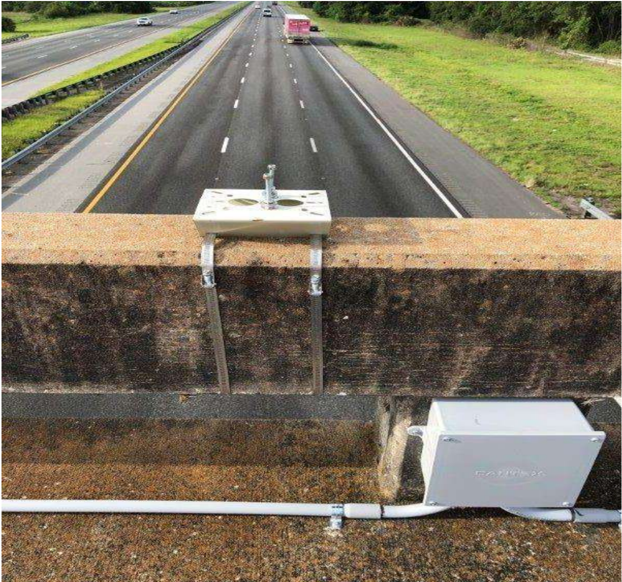
Figure 92: Bracket Ready for Capture Units
