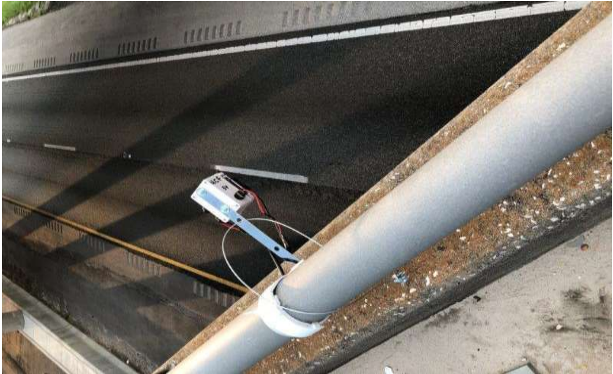
Figure 68: Capture Unit above the Highway
