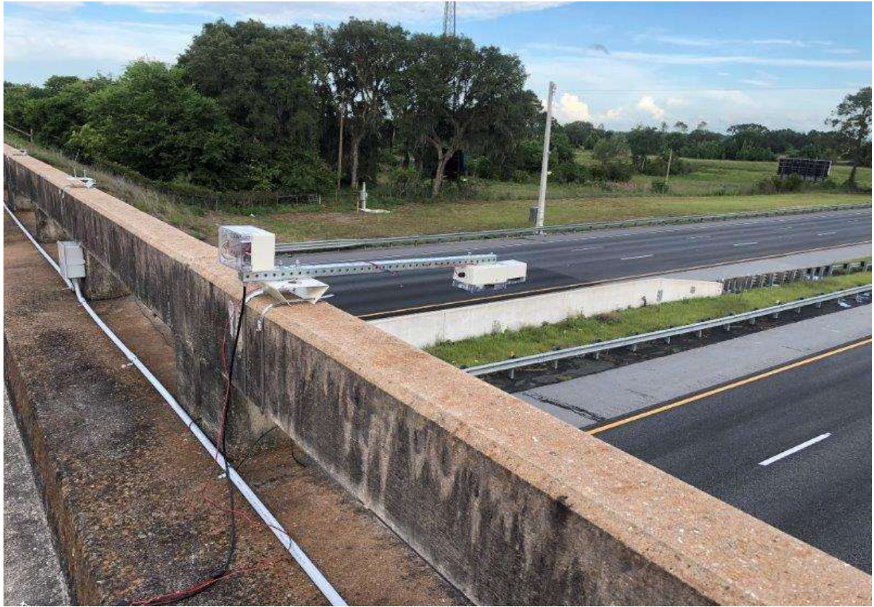
Figure 97: Site 2: Gateway Unit and Capture Unit on One Bracket
