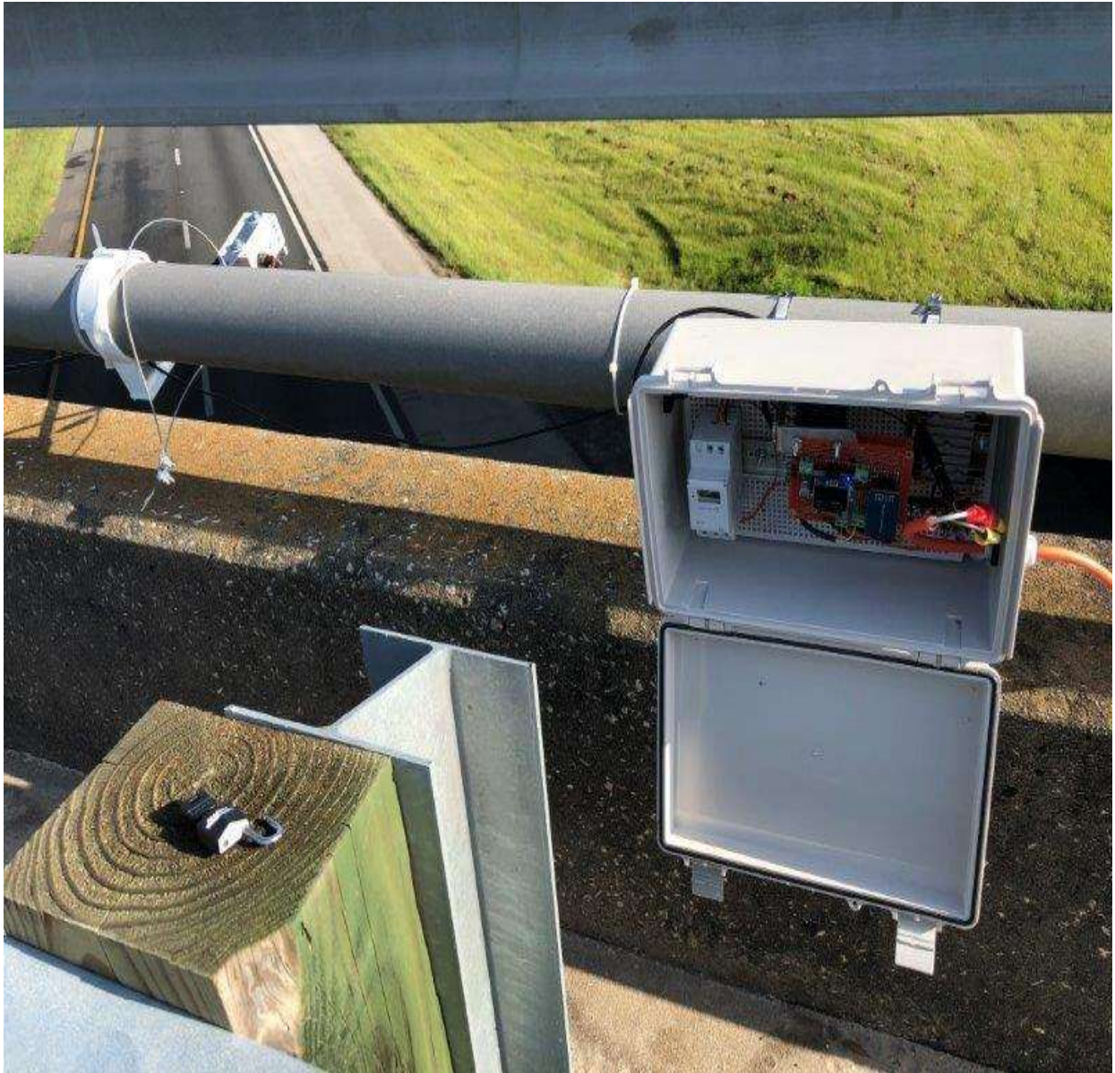
Figure 75: Gateway Board: Site 1
