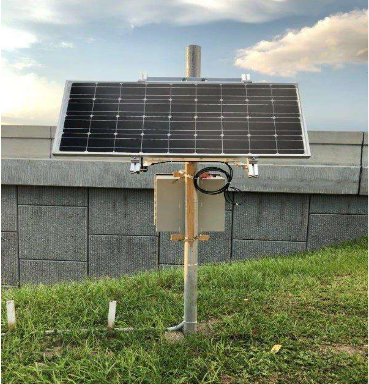
Figure 79: Solar Power Unit for Sits 1
