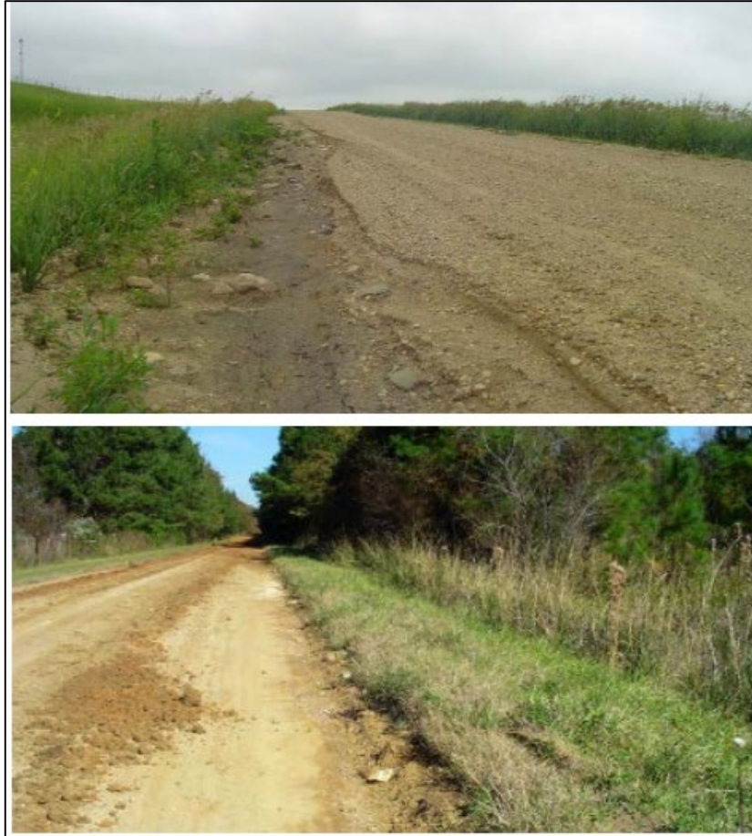
Figure 2.6 High Shoulders on road surface causing drainage issues (Federal Highway Administration, 2015)
