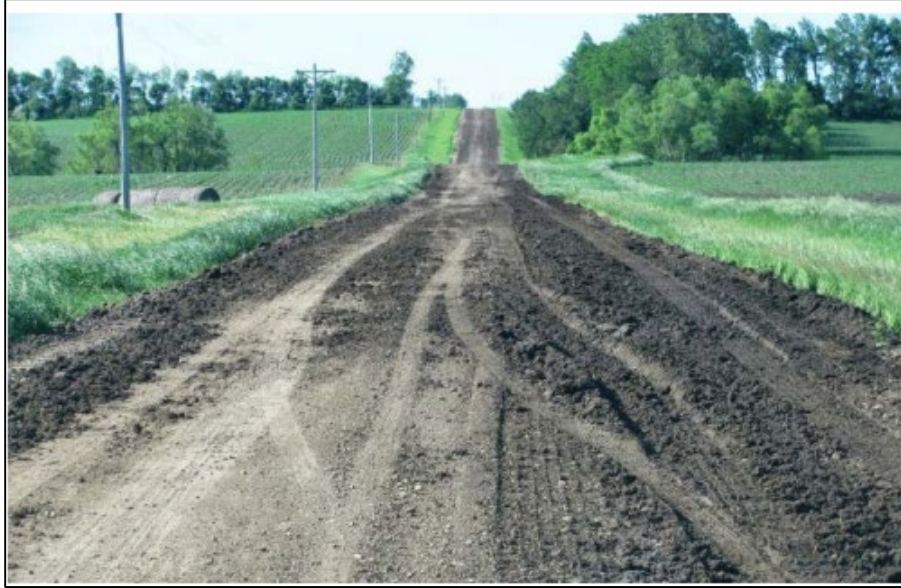
Figure 2.7 Major road deterioration (Federal Highway Administration, 2015)
