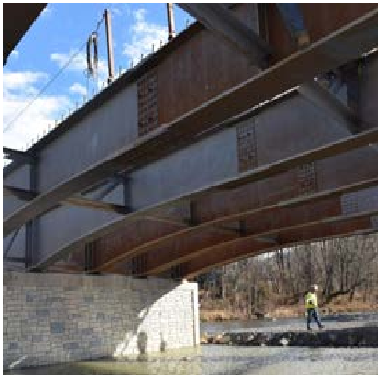
Figure 26. Various Stages of Patina on Steel Girders
