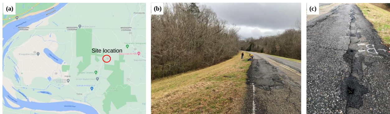
Figure 22. (a) Field test site location, (b) highway embankment slope, and (c) cracks on the highway.
