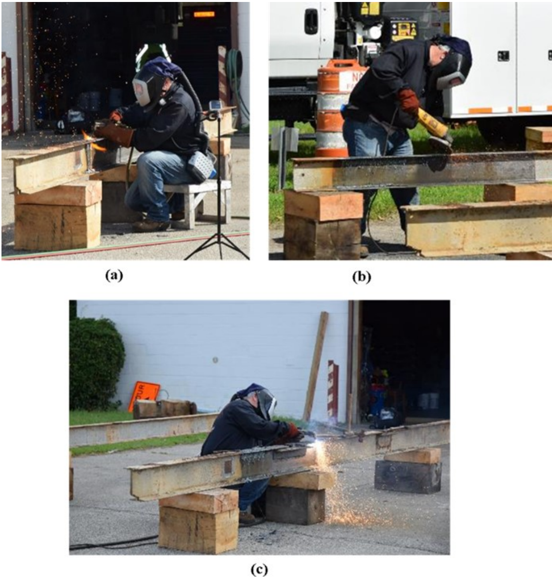
Figure 39. Various Hot Work Processes Being Performed on Beams After LACR: (a) Beam A being cut with an oxyacetylene torch in an area cleaned using LACR; (b) grinding after coating has been removed using LACR on Beam A; (c) plasma torch cutting in same cleaned area. LACR = laser ablation coating removal.
