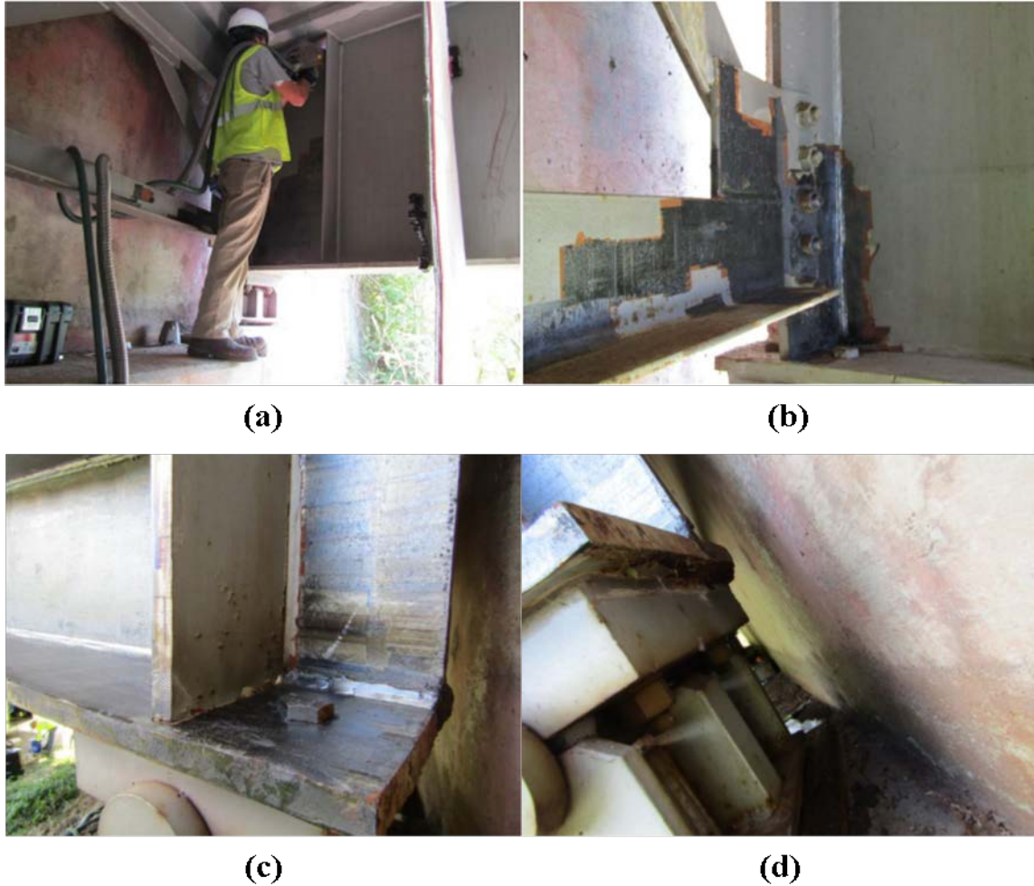
Figure 35. Laser Ablation: (a) LACR system in use to clean a component of the beam end; (b) exposed surface after laser ablation; (b, c, and d) representative images of beam ends that could not be reached with the laser for cleaning. LACR = laser ablation coating removal.
