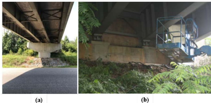
Figure 5. On-site Demonstration of LACR: (a) underside of Route 695 Bridge in Farmville, Virginia, where the on-site LACR testing took place; (b) boom lift used to elevate the operator to the cleaning area. LACR = laser ablation coating removal.
